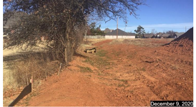
Looking north along west boundary showing upper inlet to get water into detention pond
