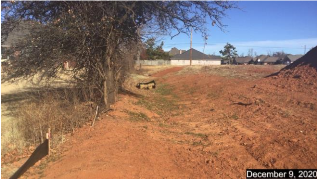
Looking north along west boundary showing upper inlet to get water into detention pond
