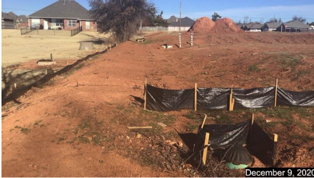
Looking north along west boundary showing inlet installed to get water into detention pond
