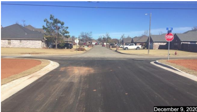
Looking north at intersection of Ryan Ridge Court / S.E. 10 th Street. Stop sign and streets signs installed. Provision for future sidewalk ramps in curb line
