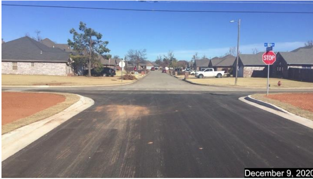
Looking north at intersection of Ryan Ridge Court / S.E. 10 th Street. Stop sign and streets signs installed. Provision for future sidewalk ramps in curb line
