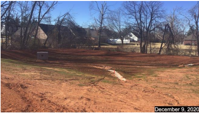
Detention pond of Ryans Ridge with paved trickle channel and weir outflow structure
