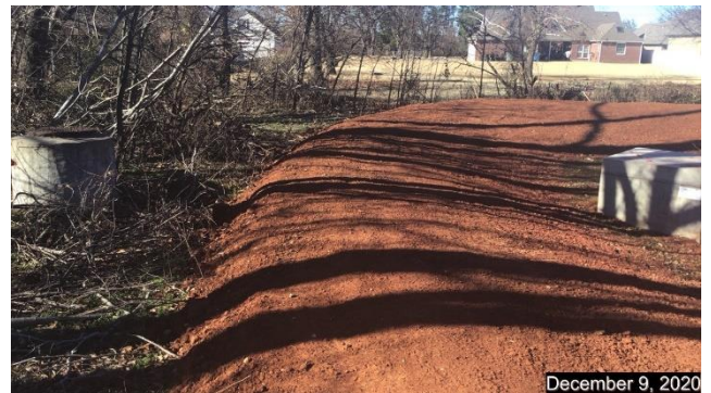
Backside of detention pond. On the right is the weir outflow structure, to the left a sanitary sewer manhole
