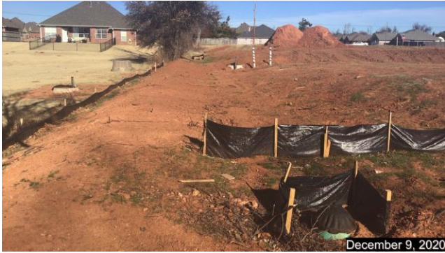
Looking north along west boundary showing inlet installed to get water into detention pond
