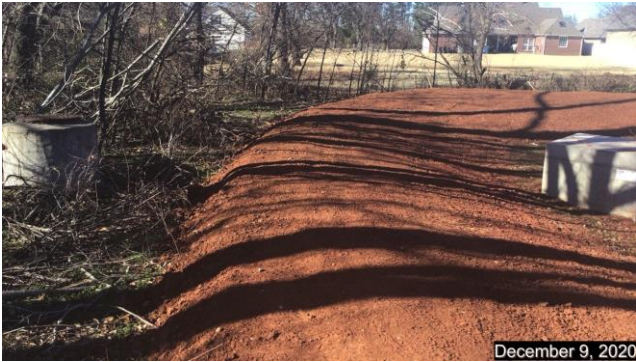
Backside of detention pond. On the right is the weir outflow structure, to the left a sanitary sewer manhole
