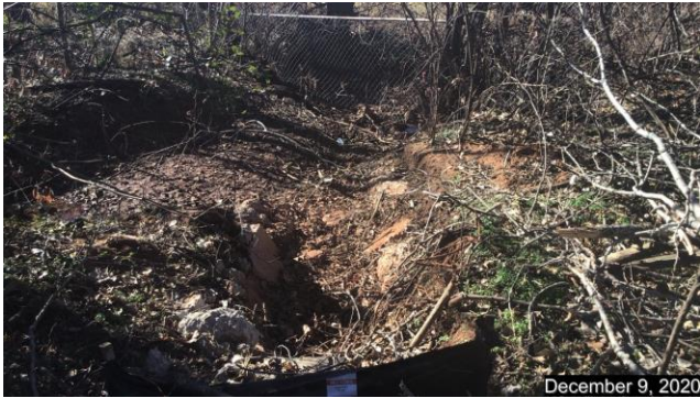
Outfall of the detention pond looking downstream of undeveloped natural drainage
