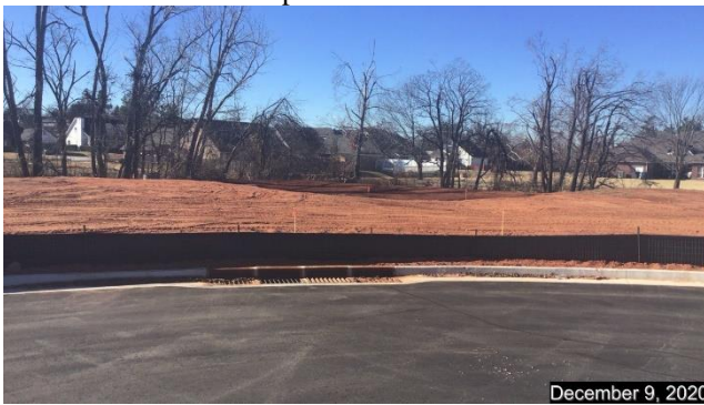
Cul-de-sac of Ryan Ridge Court, looking at inlet which flow into detention pond
