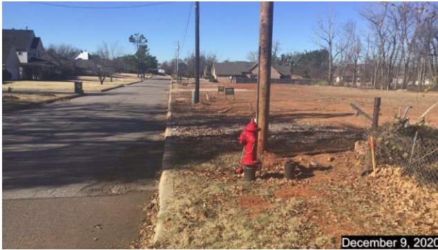
Looking west along S.E. 12 th Street, fire hydrant in foreground was installed by developer.
