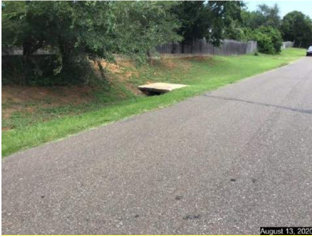
North side of SE 10 th Street, inlet catching water and taking it via 24" pipe to proposed development.
