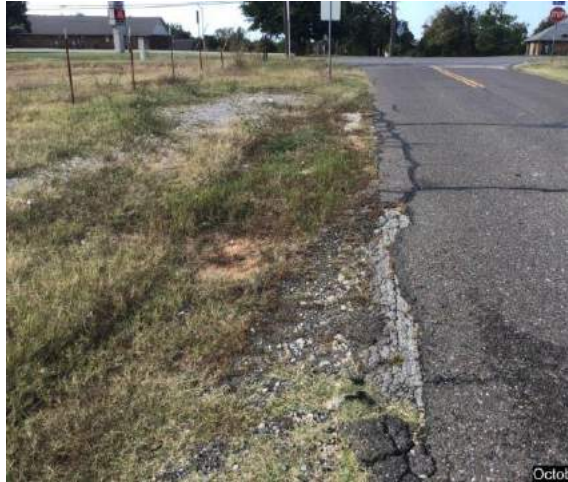
Looking west on SE 10 th Street. No Curb and Gutter or sidewalk. Note the poor condition of roadway surface.
