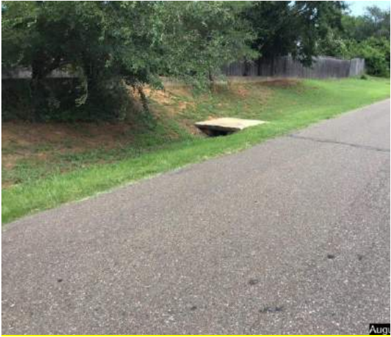
North side of SE 10 th Street, inlet catching water and taking it via 24" pipe to proposed development.
