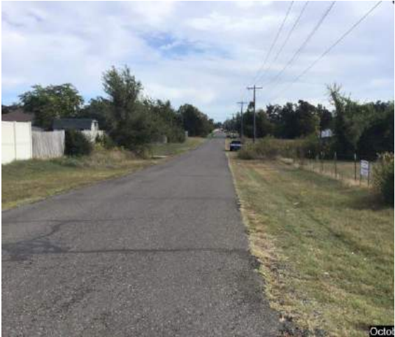
Looking east on SE 10 th Street. No Curb and Gutter or sidewalk. Note the poor condition of roadway surface.
