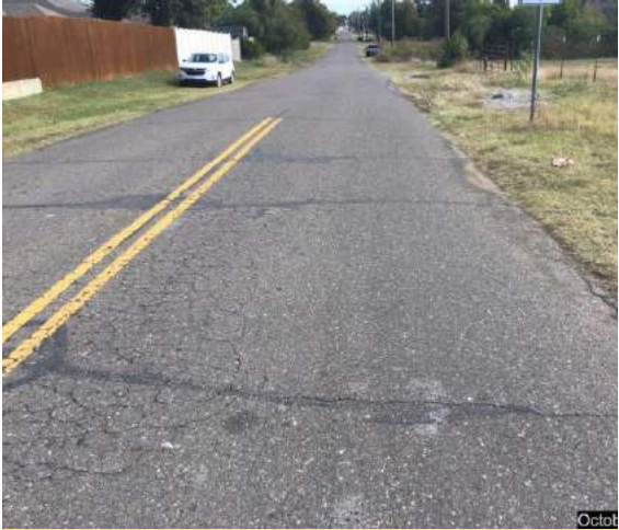
Looking east on SE 10 th Street. No Curb and Gutter or sidewalk. Note the poor condition of roadway surface.
