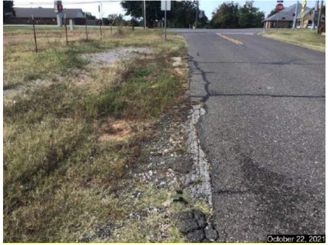
Looking west on SE 10 th Street. No Curb and Gutter or sidewalk. Note the poor condition of roadway surface.
