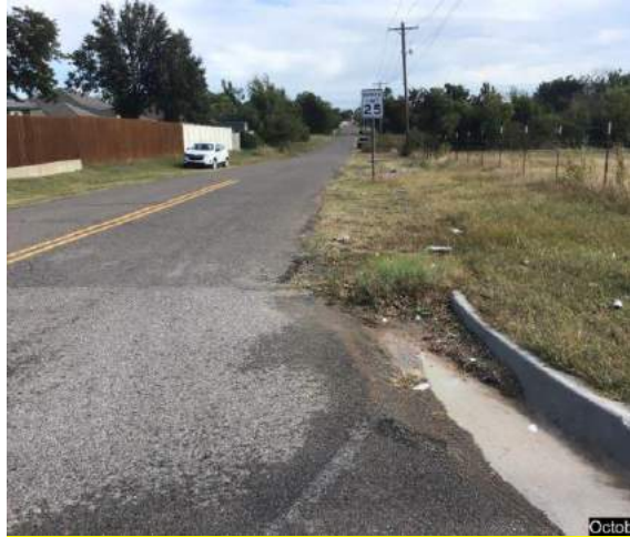
Looking east on SE 10 th Street at Post Road. Curb and Gutter from Post Road indicative of the widening required for a Collector Road.
