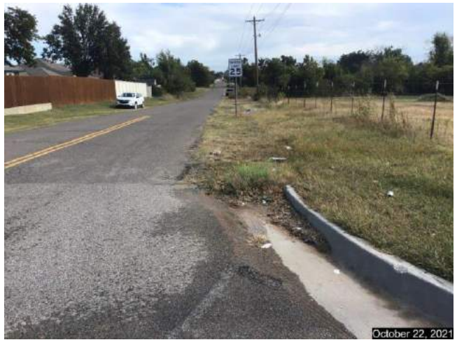
Looking east on SE 10 th Street at Post Road. Curb and Gutter from Post Road indicative of the widening required for a Collector Road.
