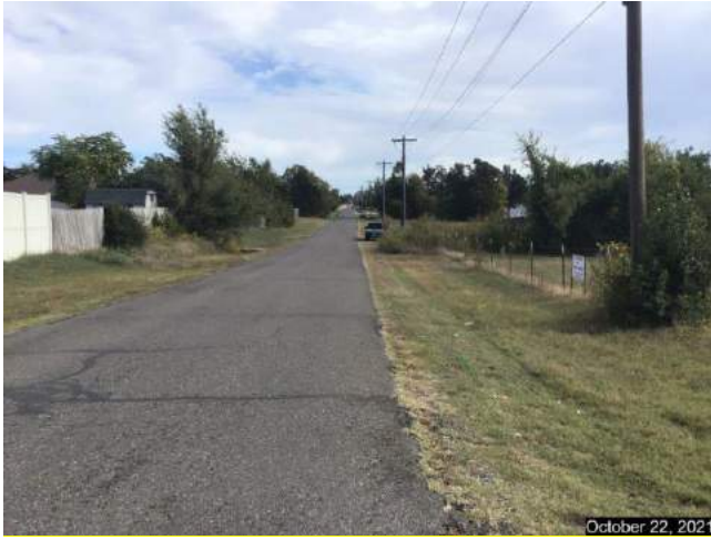
Looking east on SE 10 th Street. No Curb and Gutter or sidewalk. Note the poor condition of roadway surface.
