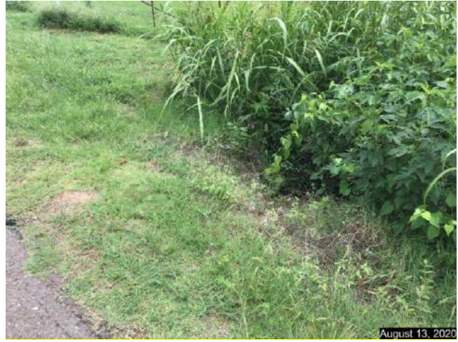
South side of SE 10 th Street, outflow of 24" cross drain opposite inlet. An inlet will need to be installed at this location.
