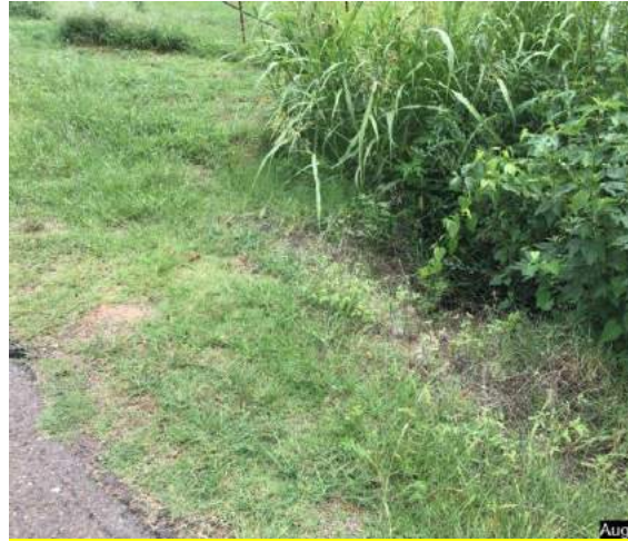
South side of SE 10 th Street, outflow of 24" cross drain opposite inlet. An inlet will need to be installed at this location.
