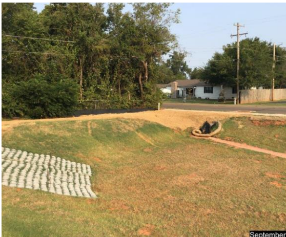
View of detention pond looking northwest. Outflow in view ties directly into existing City storm system
