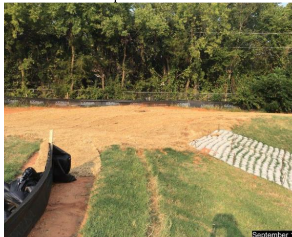
View of detention pond looking west. The area will accept sheet flow from 2 lots only with the concrete flex mat serving as scour protection.
