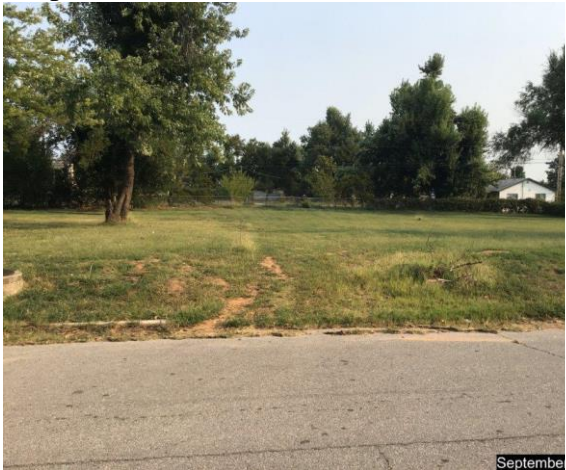
Showing curb missing. Developer would be required to repair curb as part of building permit.
