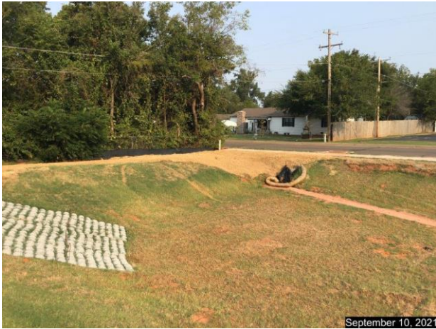
View of detention pond looking northwest. Outflow in view ties directly into existing City storm system
