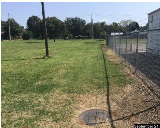
At the west property line looking east along the existing Sanitary Sewer which bisects the site
