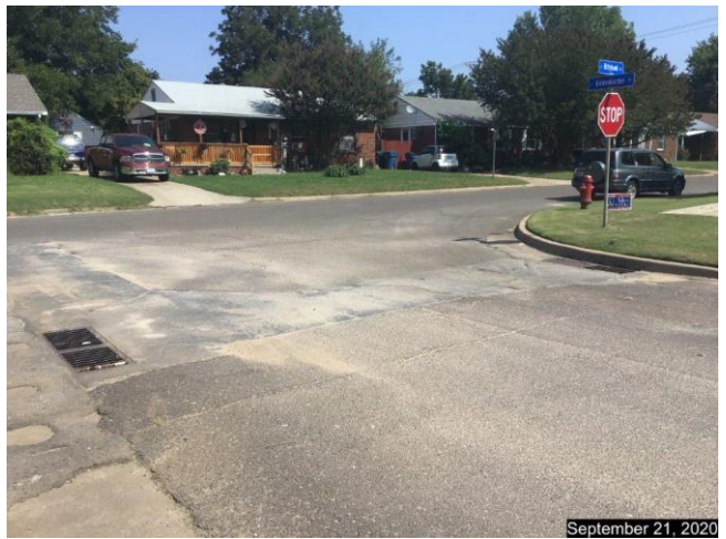
The corner of East Kittyhawk Drive and East Rickenbacker Drive. This is the upper reach of the existing drainage system. There is more infrastructure on East Kittyhawk Drive just downstream (to the west) of this intersection.
