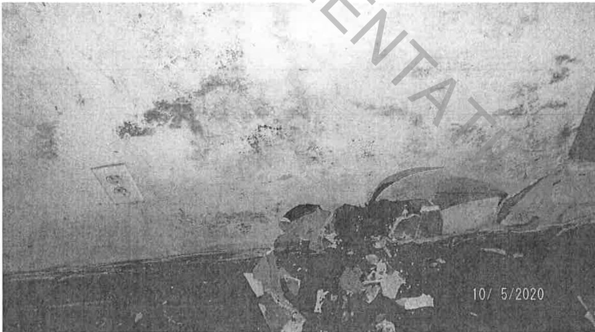
Photo B: Typical mold throughout
