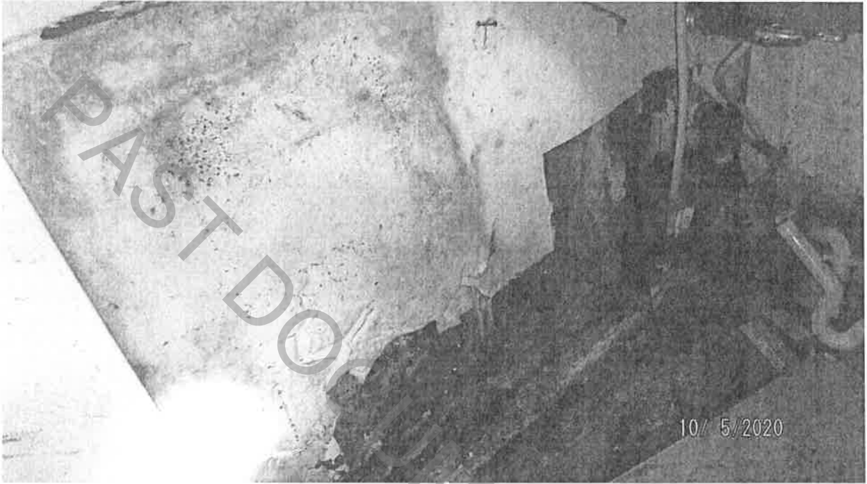
Photo A: Mold on kitchen wall
