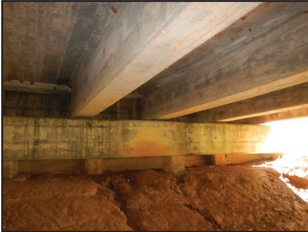
Photo 11. Erosion and Exposed Piles at East Abutment
