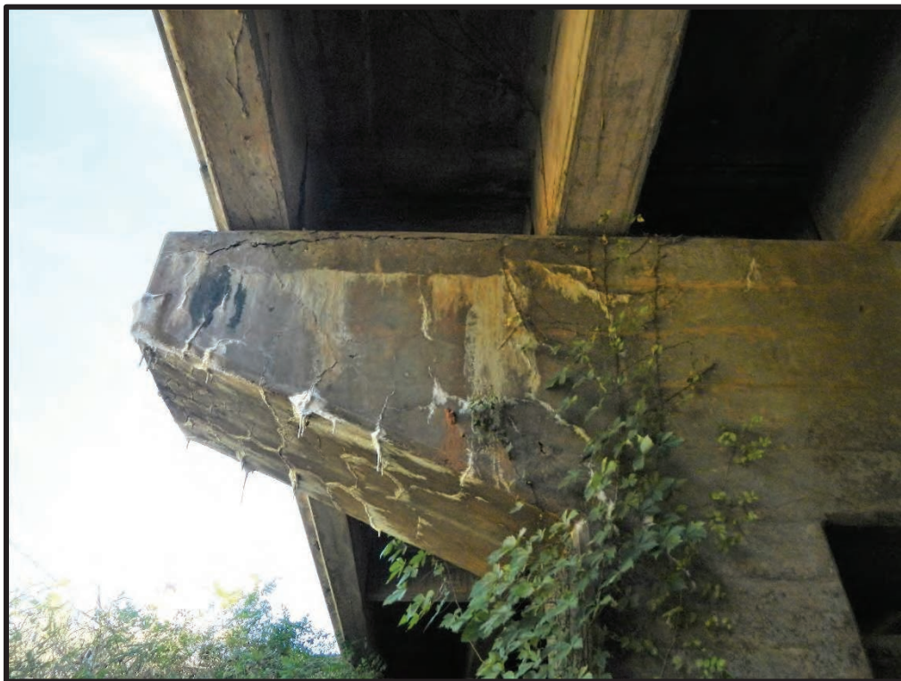
Photo 15. Pier Cap Leaching and Cracking
