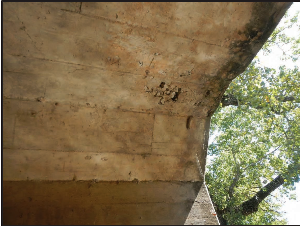
Photo 31. Honeycombing at South End of Barrel
