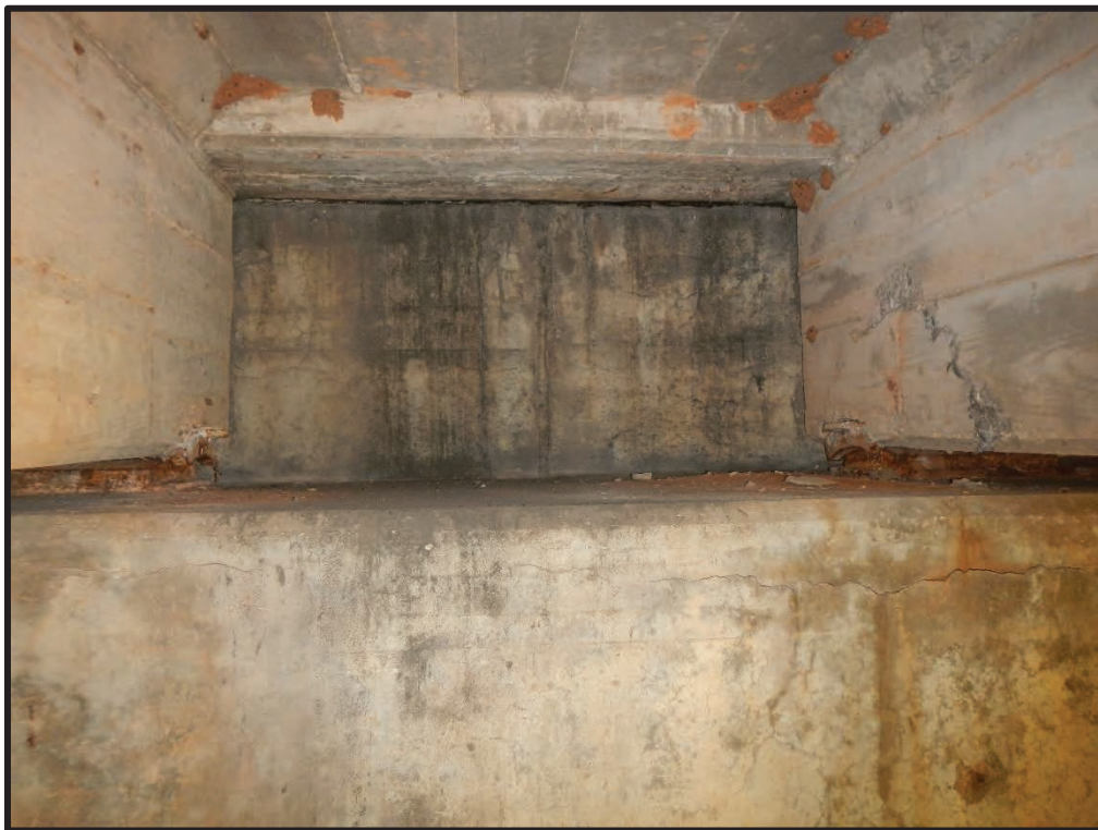
Photo 10. Abutment Discoloration and Cracking
