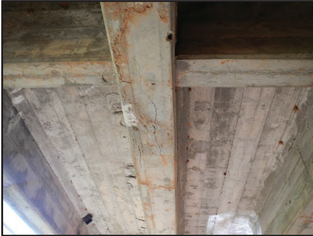
Photo 21. Typical Cracking in Girder Bottom
