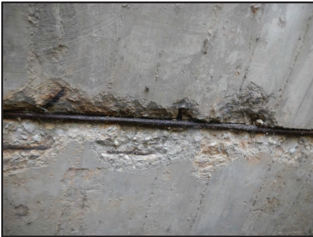
Photo 38. Close Up of Exposed Rebar at Construction Joint
