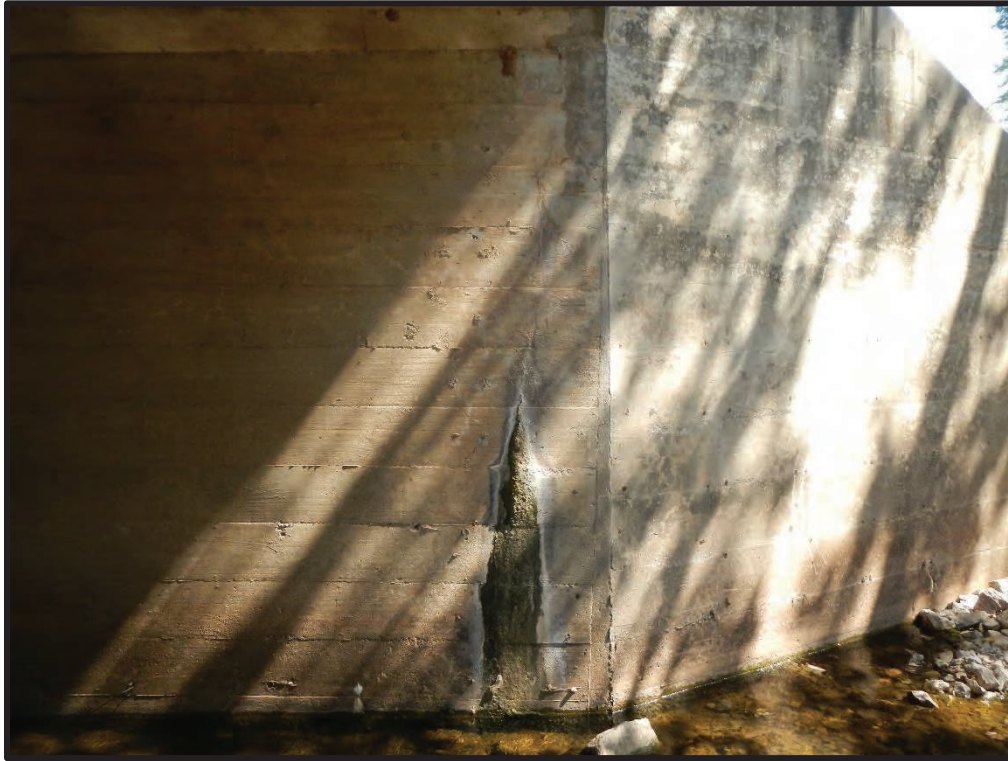
Photo 35. Wing Connection Cracking and Leaching
