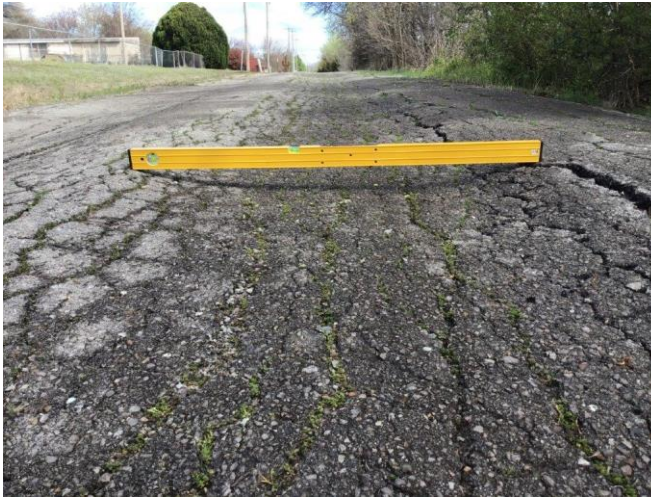
Looking north on Davidson Drive, east side of roadway. Note the presence of rutting and alligator cracking.
