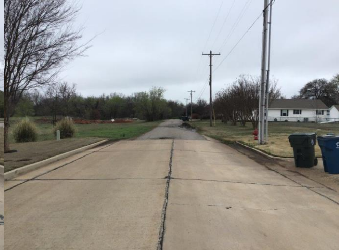
Looking south on Davidson Dr. Development area on west side of street.
