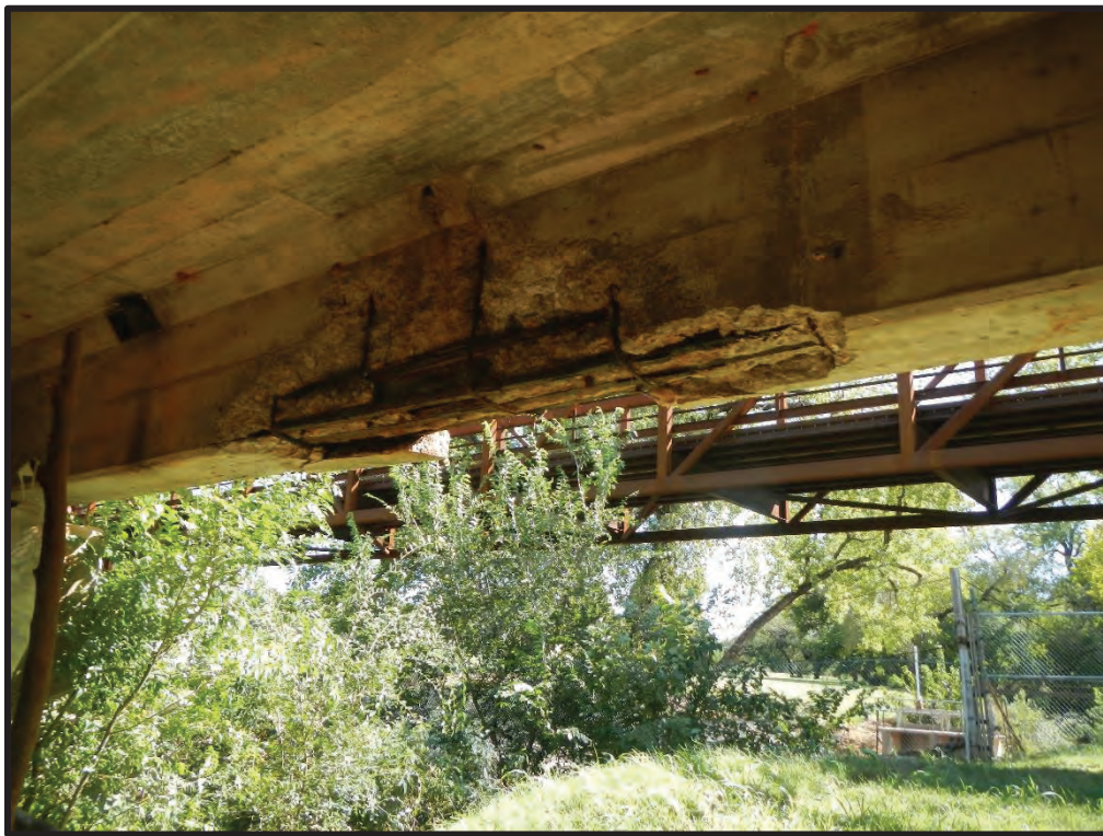
Photo 20. Severe Spalling and Rebar Corrosion
