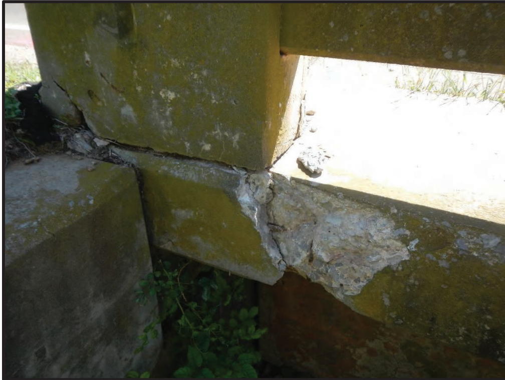
Photo 6. Typical Spalling at Concrete Curb
