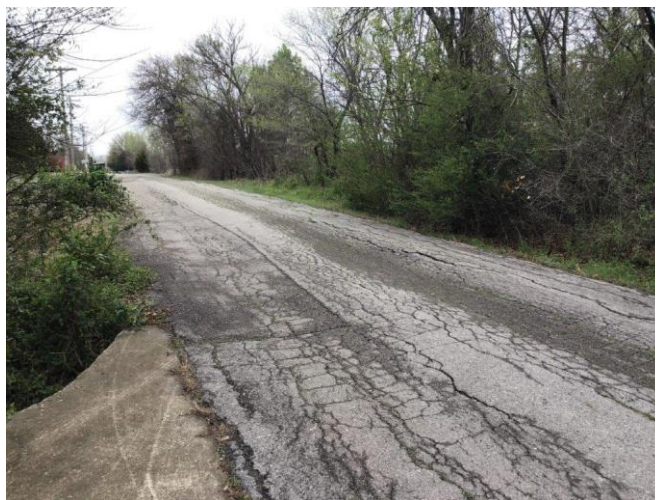
Looking north from end of Davidson Drive. Note condition of roadway
