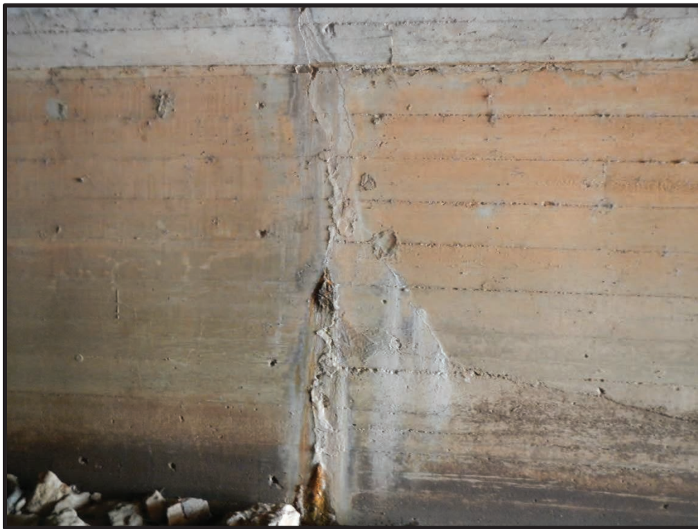
Photo 36. Typical Leaching at Construction Joint
