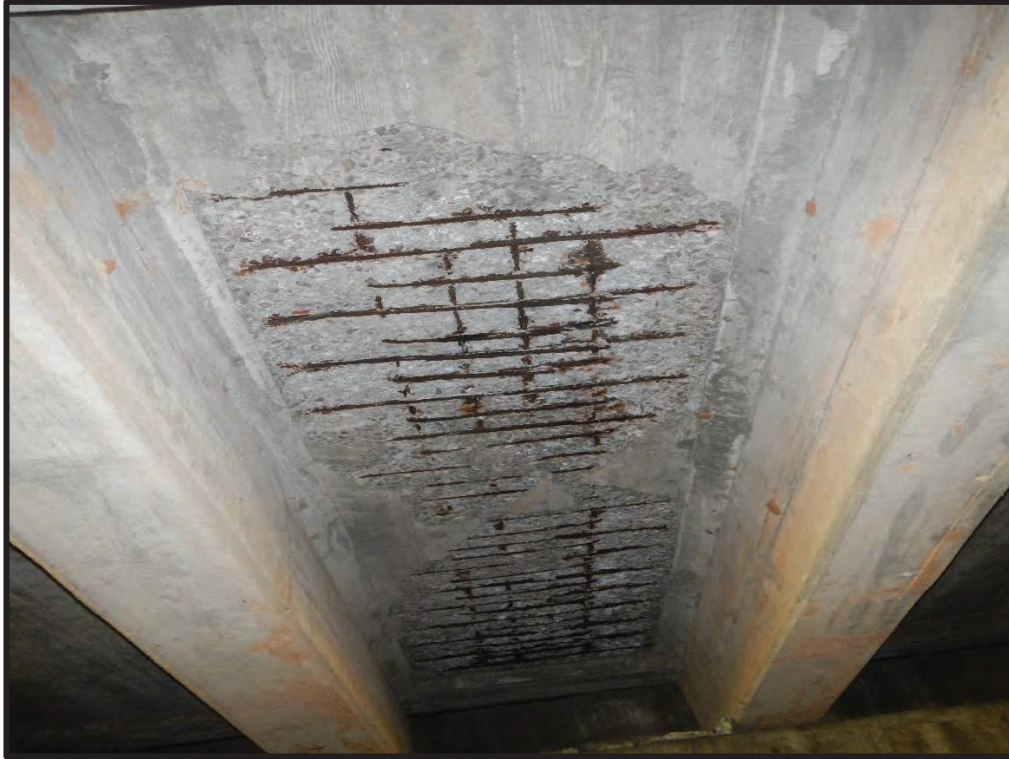
Photo 23. Spalling in Deck Soffit with Exposed Rebar
