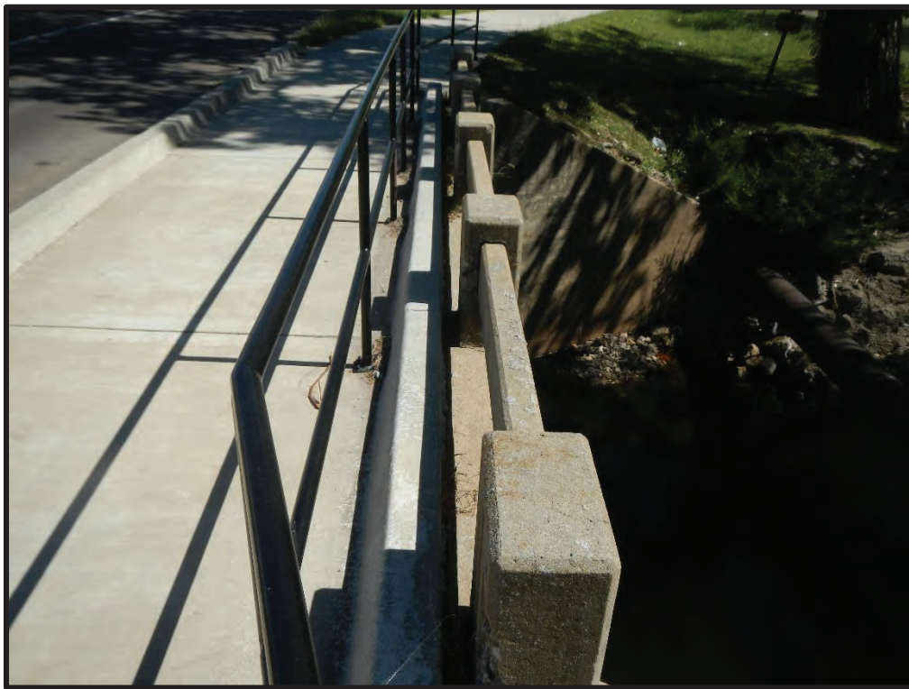
Photo 28. Typical Condition of Concrete Traffic Rail
