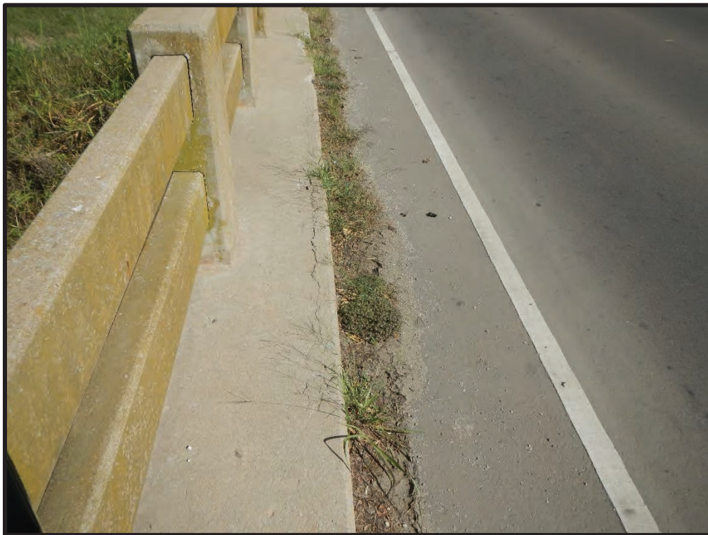
Photo 7. Cracking at Curb and Vegetation
