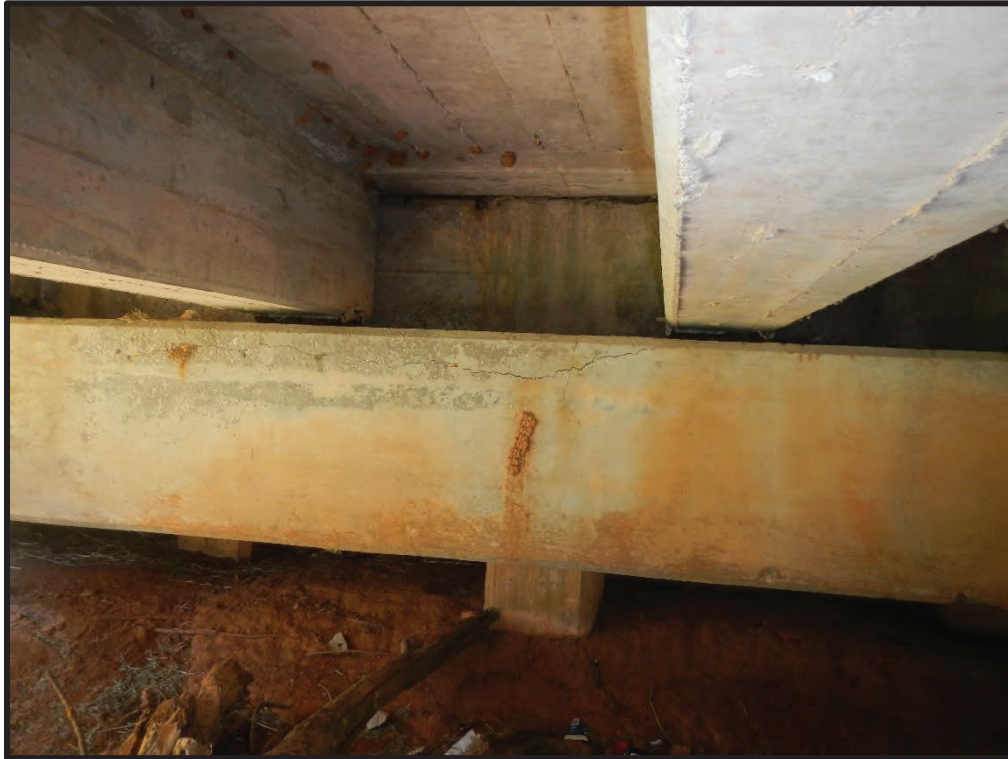
Photo 9. Abutment Seat Cracking and Exposed Piles
