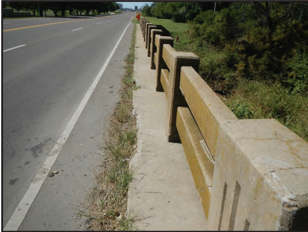
Photo 4. Typical Condition of Concrete Traffic Rail and Vegetation along Curb
