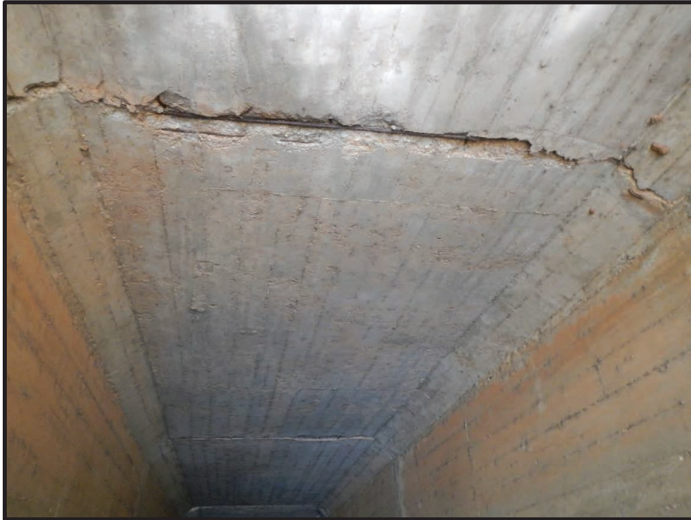
Photo 37. Typical Spalling and Exposed Rebar at Top Construction Joint
