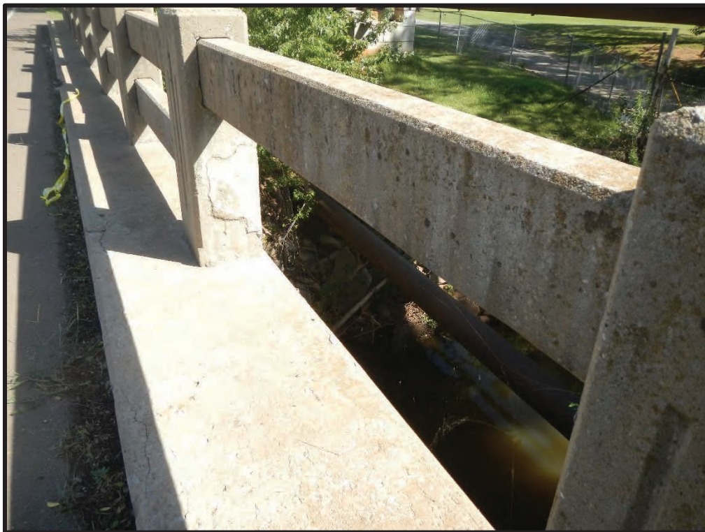
Photo 5. Missing Bottom Rail
