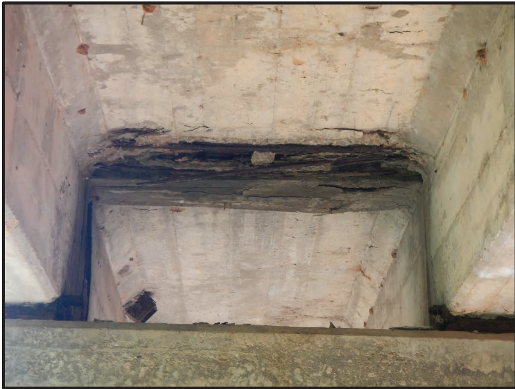
Photo 24. Typical Spalling and Corroded Rebar at Pier
