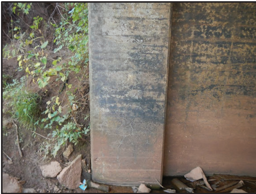
Photo 17. Typical Pier Column Map Cracking
