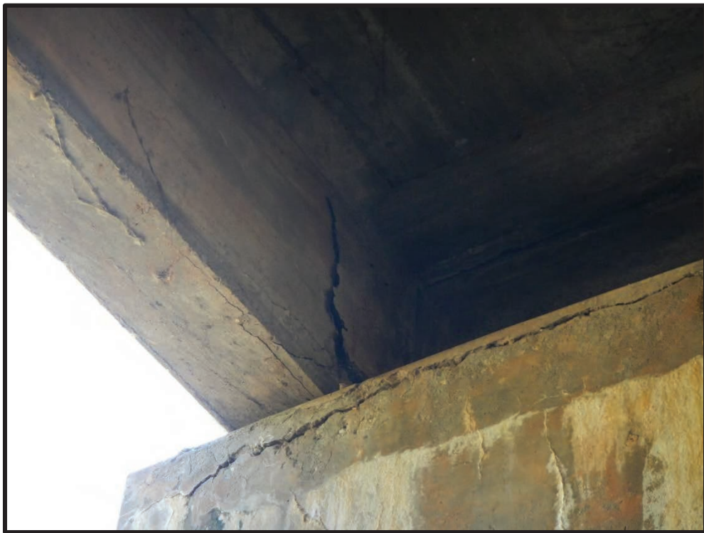
Photo 18. Cracking and Delamination at Girder-End
