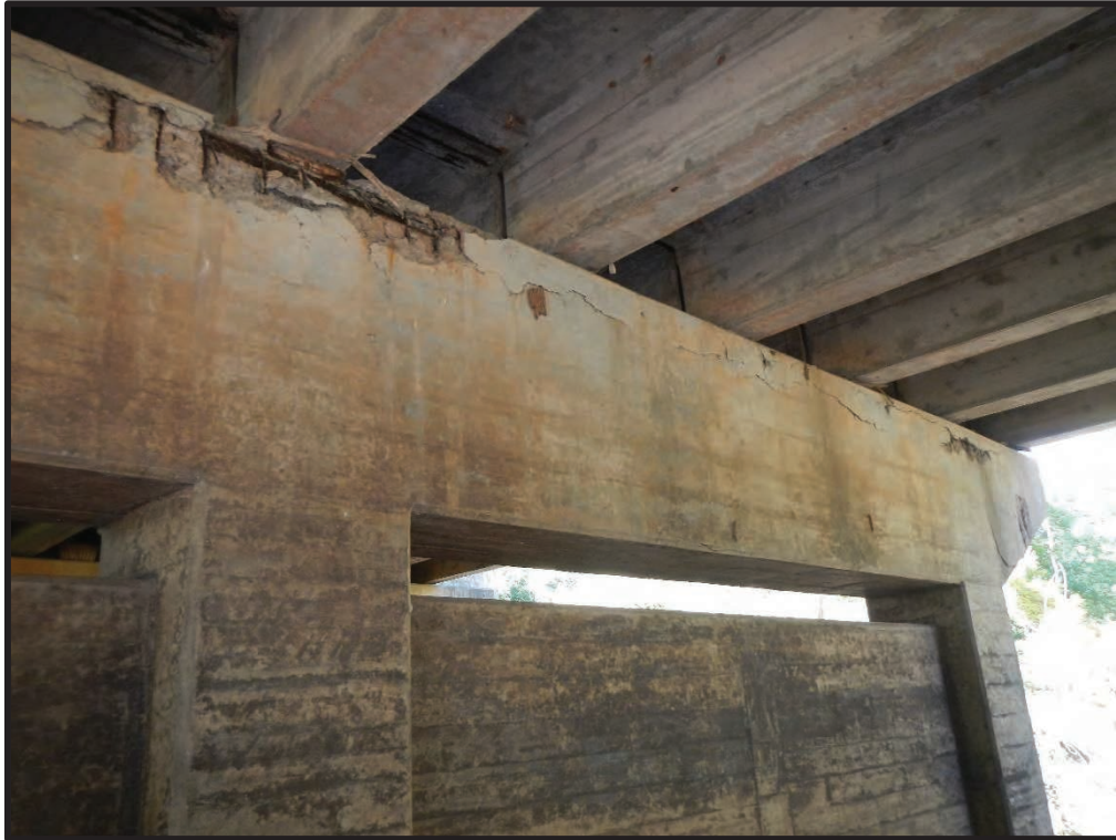
Photo 14. Pier Cap Cracking, Spalling and Rebar Corrosion
