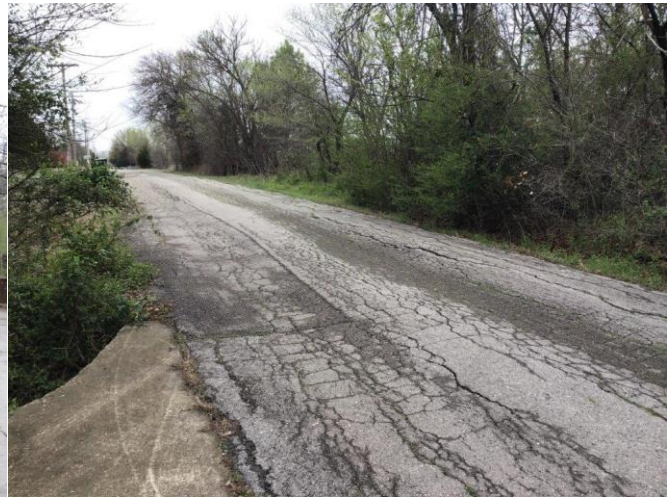
Looking north from end of Davidson Drive. Note condition of roadway.
