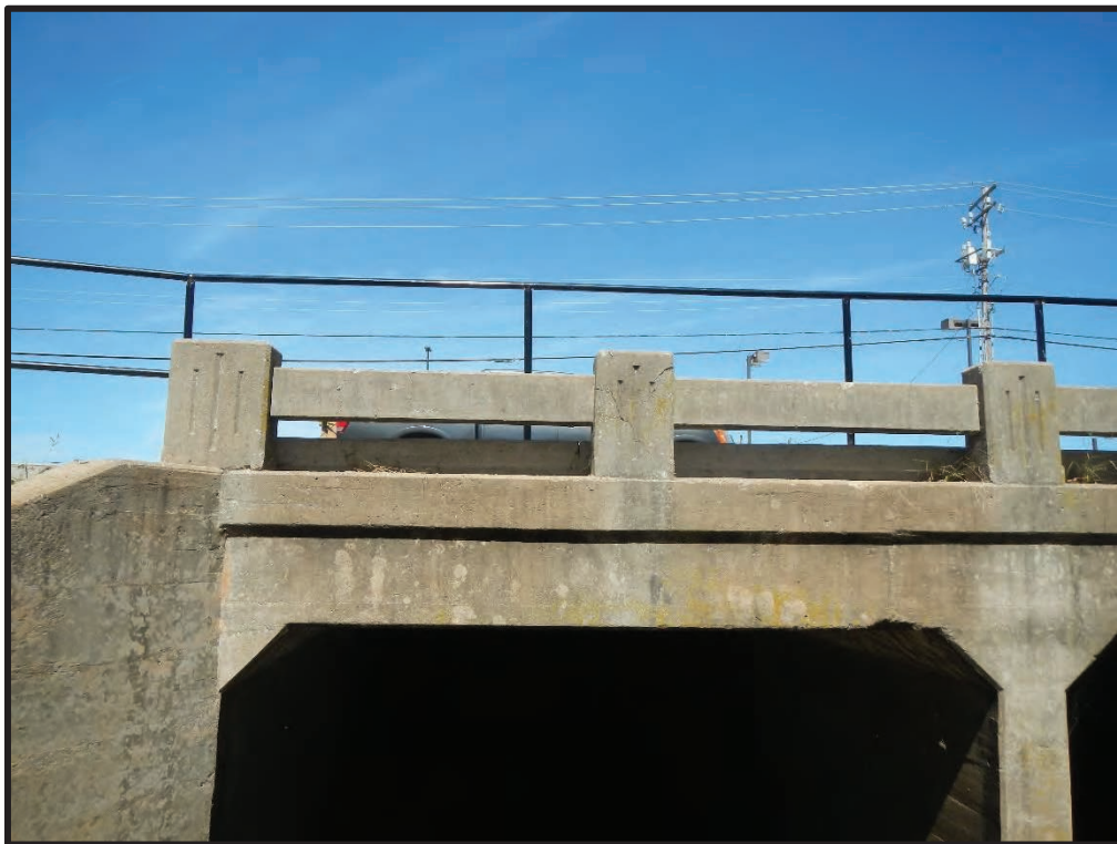
Photo 30. Typical Condition of Head Wall and Concrete Traffic Rail
