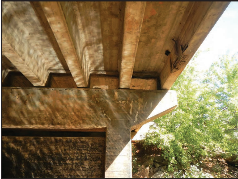
Photo 16. Typical Cracking at Pier Cap
