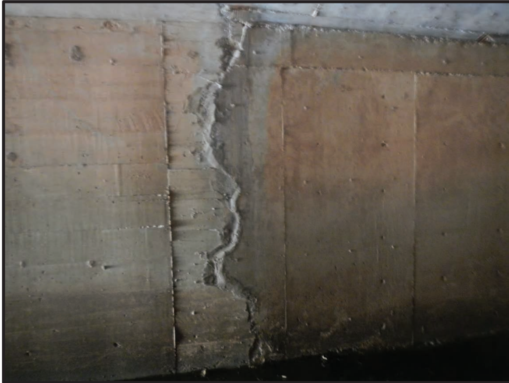
Photo 39. Cracking at Construction Joint
