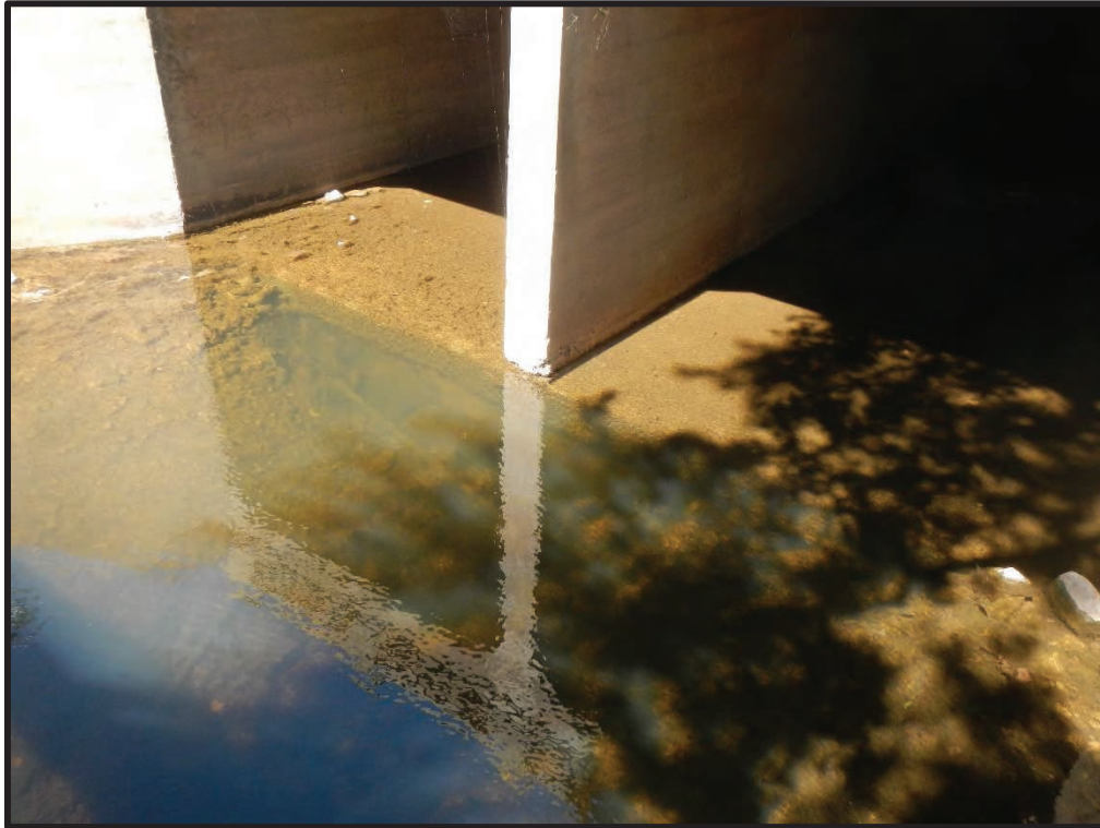
Photo 33. Scour Hole at Inlet
