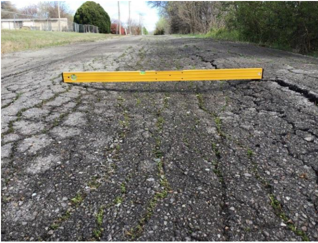
Looking north on Davidson Drive, east side of roadway. Note the presence of rutting and alligator cracking.
