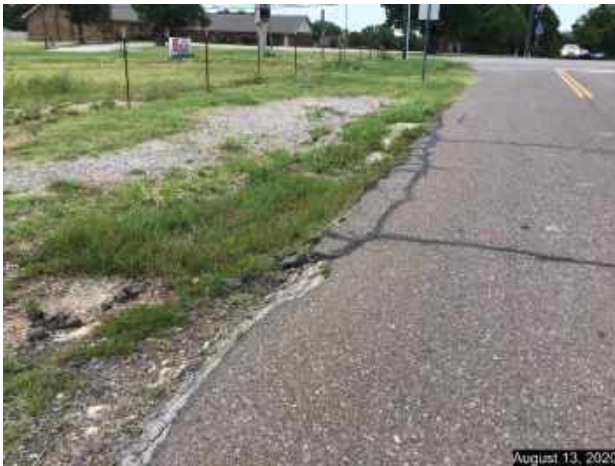
Looking west on SE 10 th Street. No Curb and Gutter or sidewalk. Note the poor condition of roadway surface.
