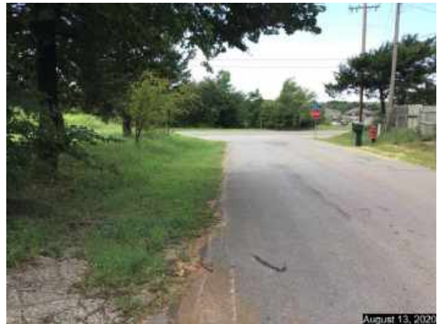
Looking west on SE 28 th Street. No Curb and Gutter or sidewalk. Note the poor condition of roadway surface.
