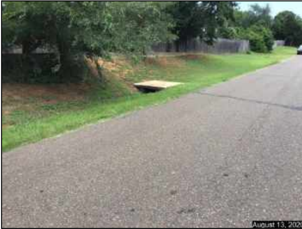
North side of SE 10 th Street, inlet catching water and taking it via 24" pipe to east side of property in question.
