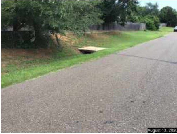
North side of SE 10 th Street, inlet catching water and taking it via 24" pipe to east side of property in question.
