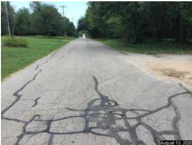
Looking east on SE 28 th Street. No Curb and Gutter or sidewalk. Note the poor condition of roadway surface.
