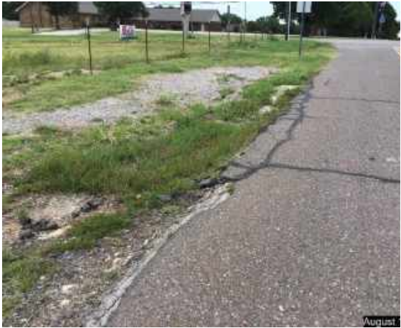
Looking west on SE 10 th Street. No Curb and Gutter or sidewalk. Note the poor condition of roadway surface.
