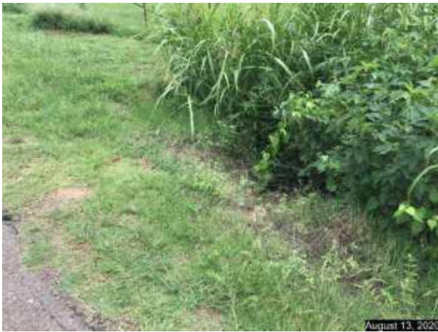
South side of SE 10 th Street, outflow of 24" cross drain opposite inlet.
