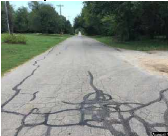
Looking east on SE 28 th Street. No Curb and Gutter or sidewalk. Note the poor condition of roadway surface.
