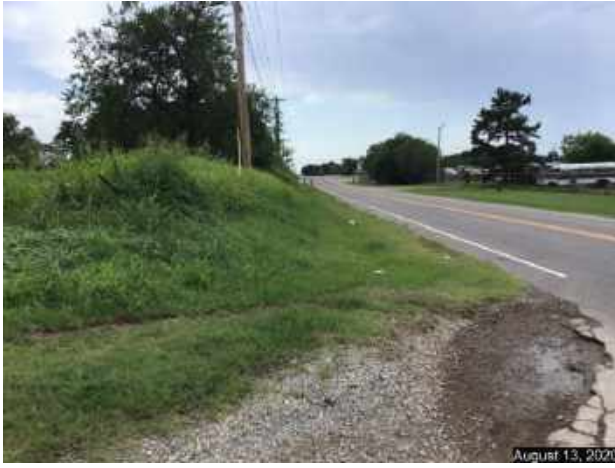
Looking south at corner of SE 28 th Street and Westminster Road. No Curb and Gutter or sidewalk. Note the poor condition of roadway surface.
