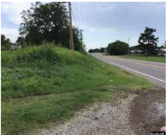
Looking south at corner of SE 28 th Street and Westminster Road. No Curb and Gutter or sidewalk. Note the poor condition of roadway surface.
