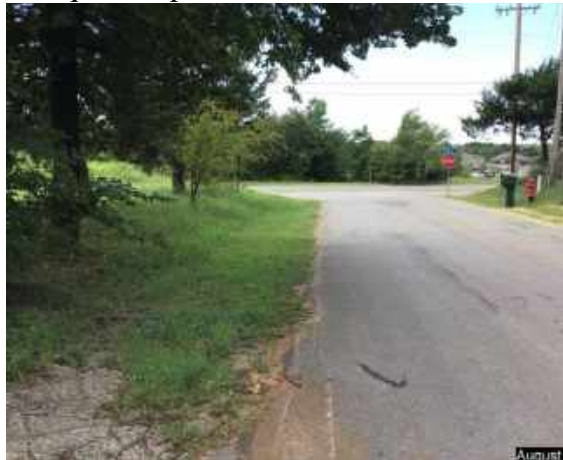
Looking west on SE 28 th Street. No Curb and Gutter or sidewalk. Note the poor condition of roadway surface.
