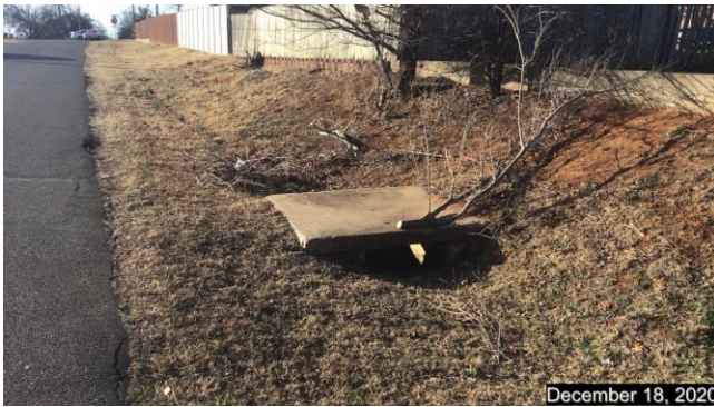
Drainage inlet on north side of S.E. 10 th Street which drains to the south
