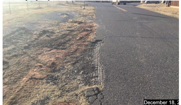
S.E. 10 th Street, note the top layer of asphalt separated from underlying road.
