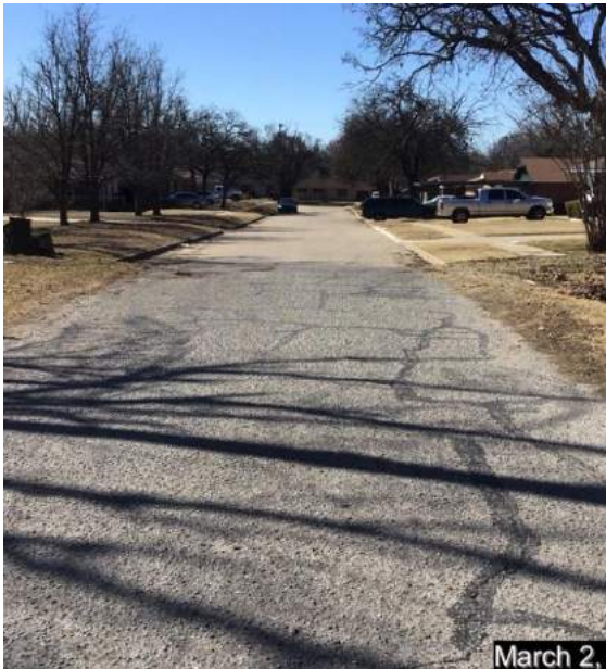
Looking west from western edge of subject plat. Shows NE 5 th Street in a city standard configuration. Concrete with curb and gutter on both sides and sidewalk
