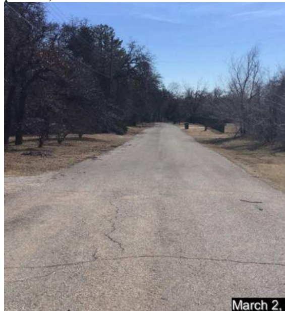
Looking south from intersection of NE 5 th Street and Oakview Drive along Oakview Drive showing substandard street. Subject plat is on the west side (right of picture)
