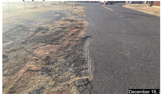
S.E. 10 th Street, note the top layer of asphalt separated from underlying road.
