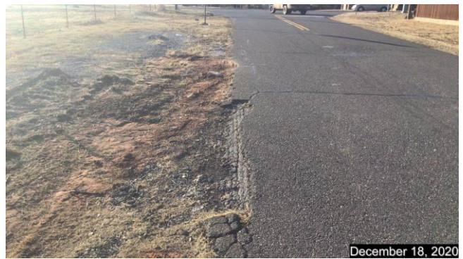
S.E. 10 th Street, note the top layer of asphalt separated from underlying road.
