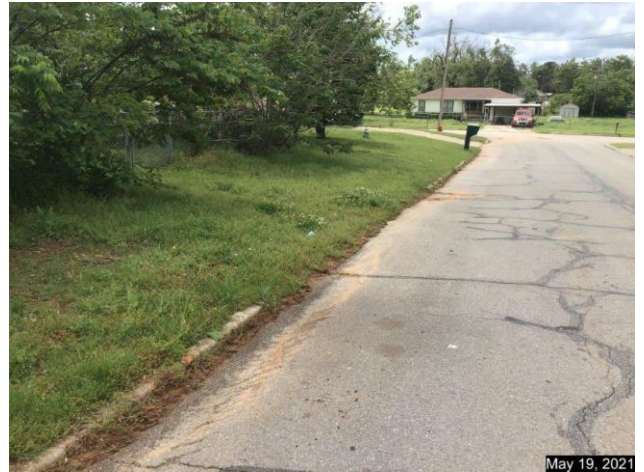
Showing curb missing. Developer would be required to repair curb as part of building permit.
