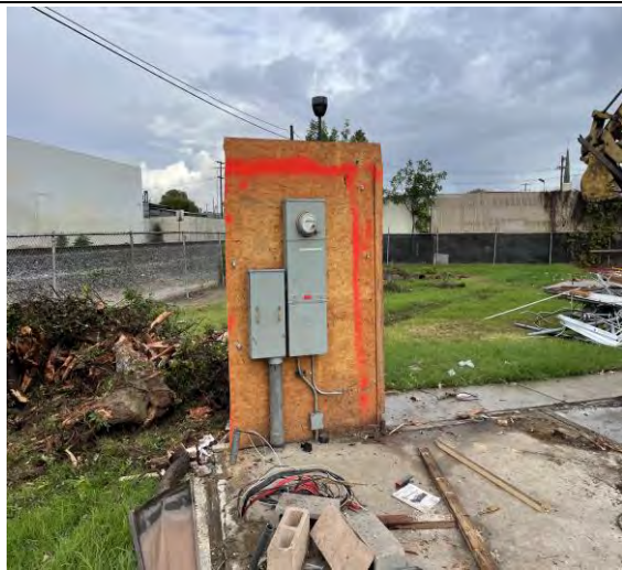
Existing Electrical Panel to be deenergized prior to demolition
