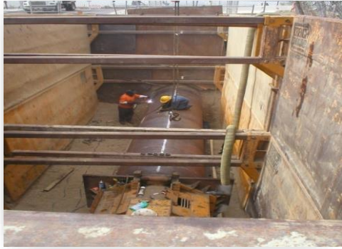
Figure 1. We thrive in creating solutions to challenging problems. The 1720 Zone West project required deep pit bore and jack construction under an active freight rail line, requiring significant permitting efforts and additional construction coordination.
