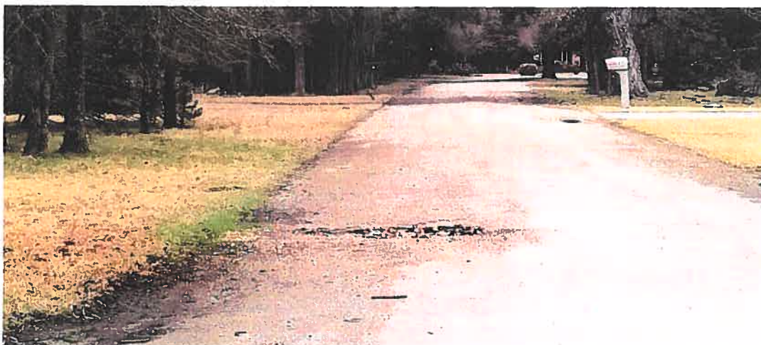
Figure 10. Pothole on Buckeye Court
