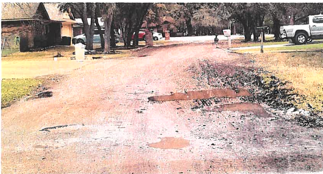
Figure 8. Potholes on Basswood Court
