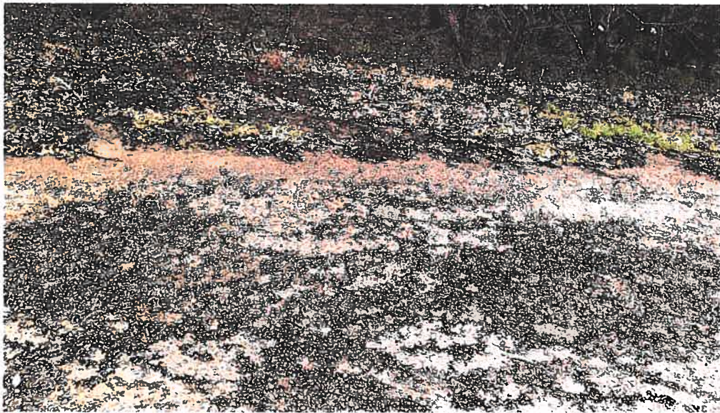
Figure 4. Alligator Cracks on Canyon Circle
