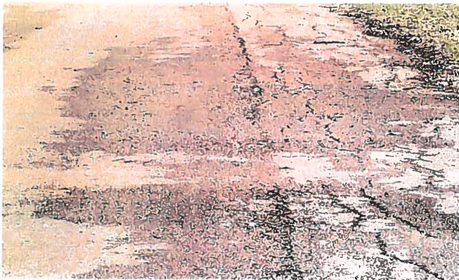
Figure 16. Alligator Cracks on Buckskin Loop
