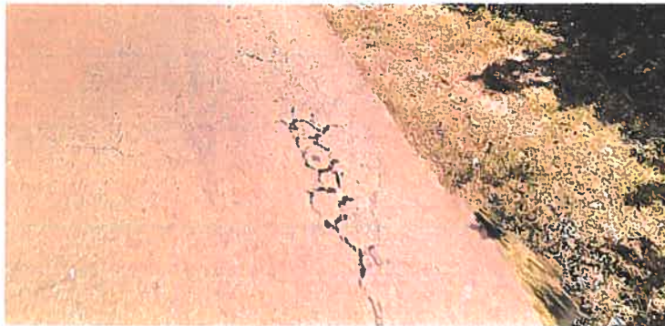
Figure 14. Cracks on Lake Forest Drive
