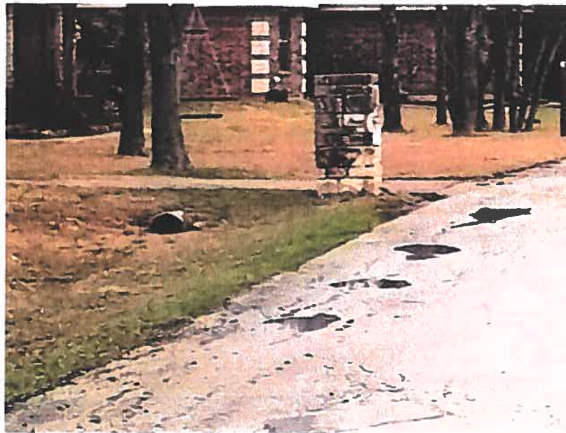
Figure 12. Potholes on Shetland Drive
