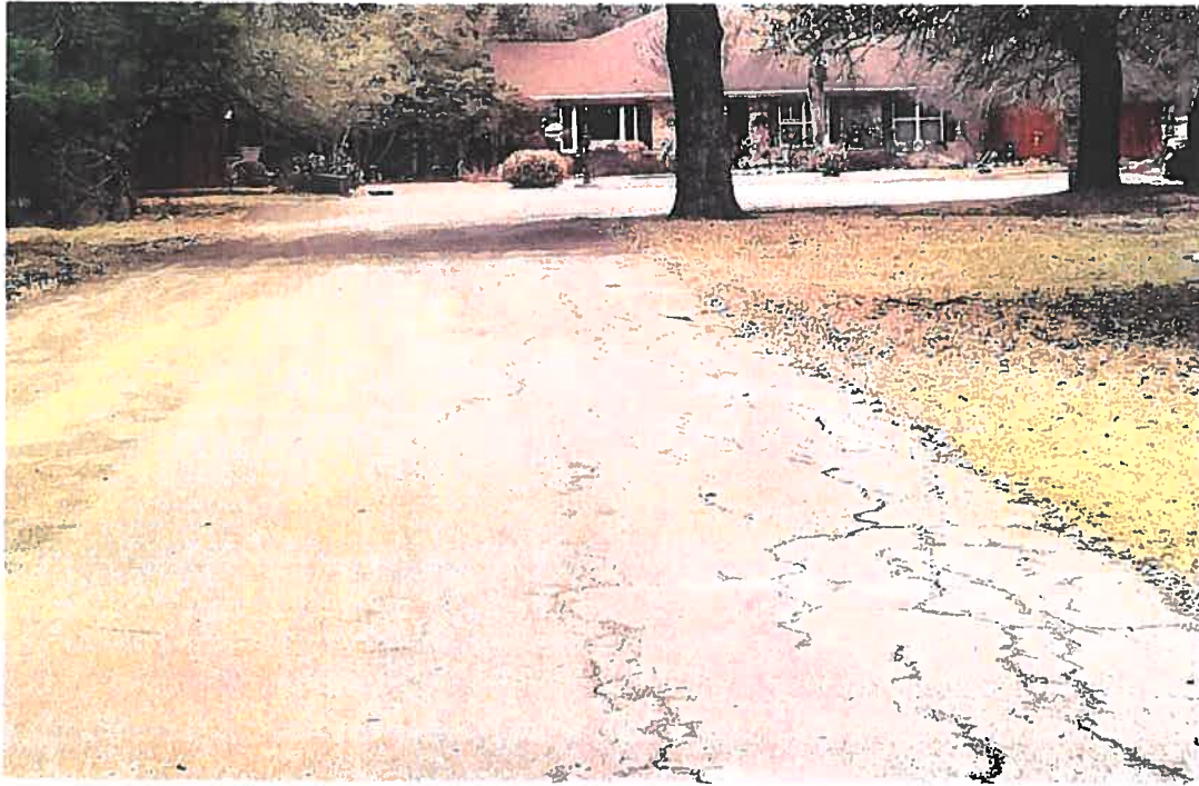
Figure 11. Alligator Cracks on Buckeye Court
