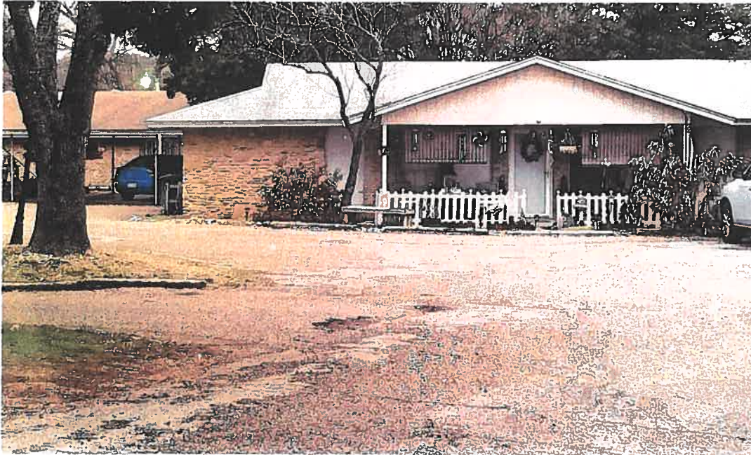
Figure 17. Pavement Condition for Mariner Drive
