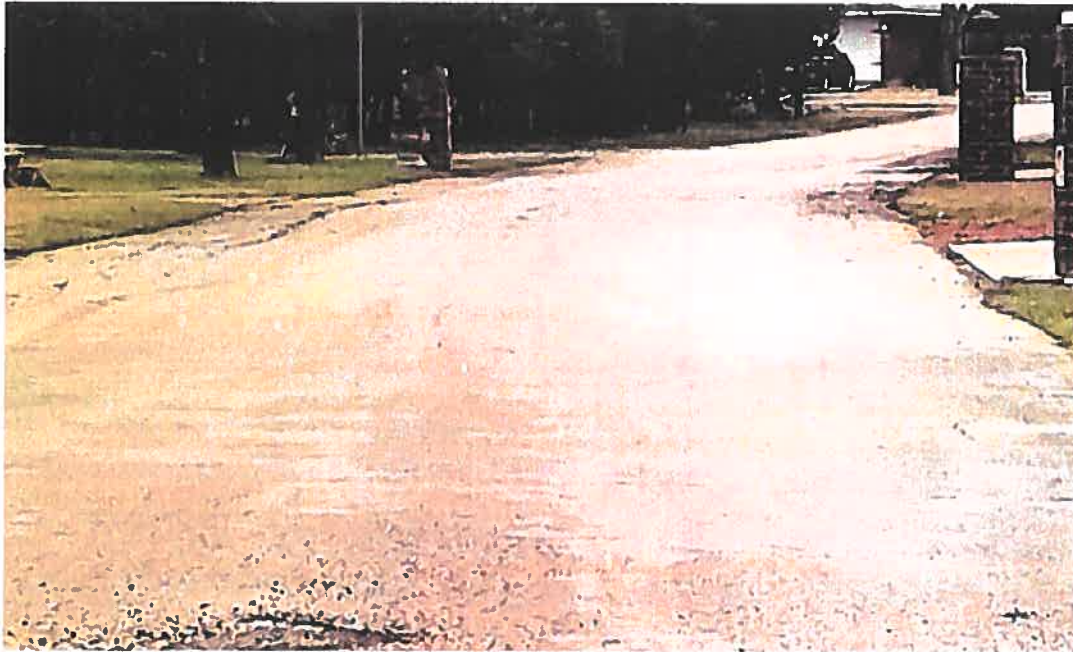
Figure 13. Alligator Cracks on Shetland Drive
