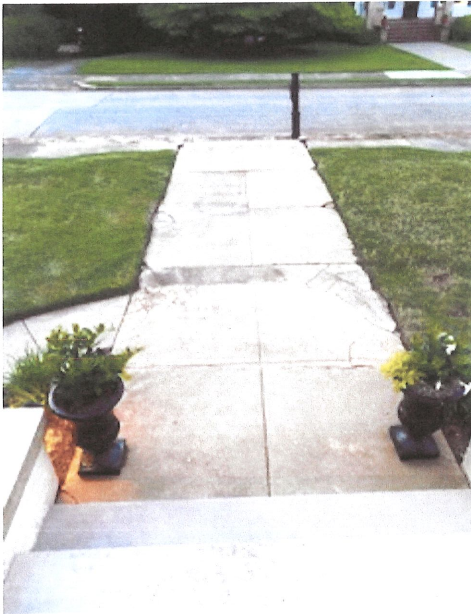
Sidewalk from house to street Broken in many areas
