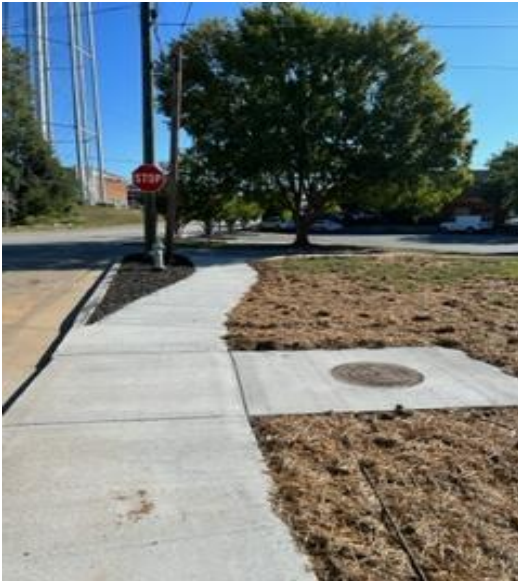
400 feet of sidewalk along W. Washington Street leading into Childers Park was replaced using a combination of contract and City labor.
