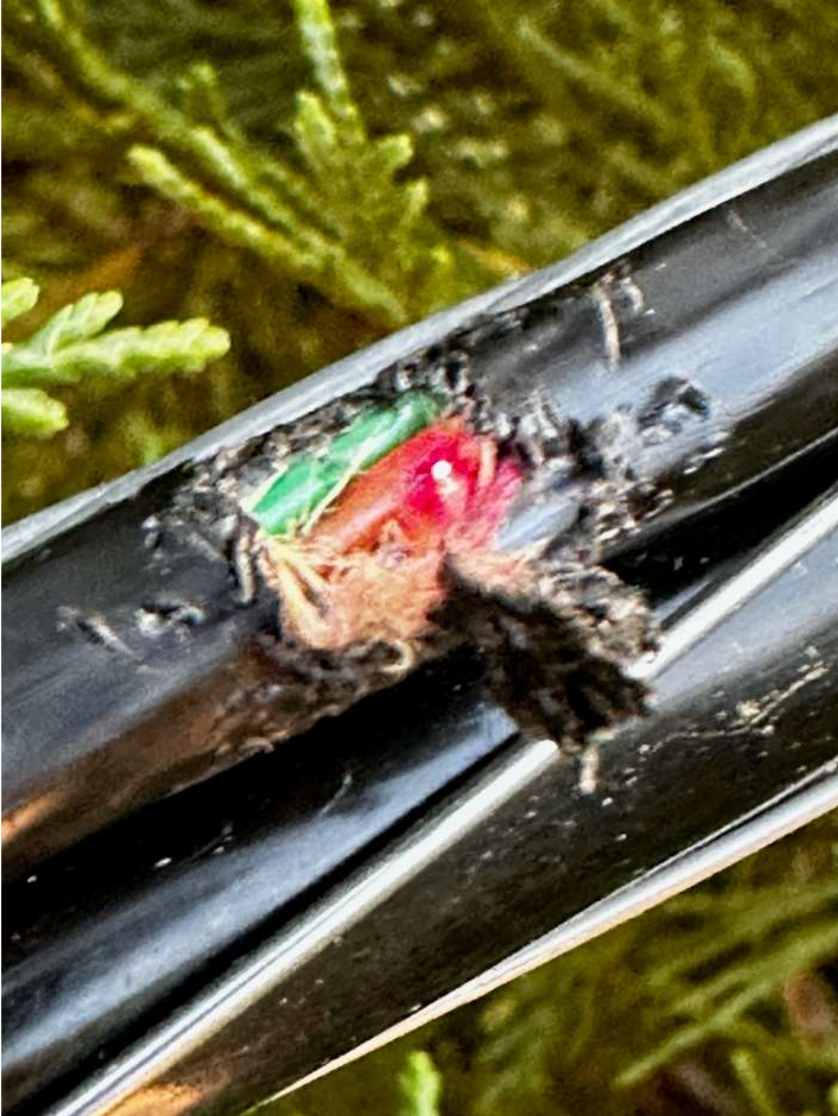
A single squirrel chew in a 30+ mile fiber route that had to be located and repaired. This incident occurred twice in the month of April and both times required several hours of repair time.
