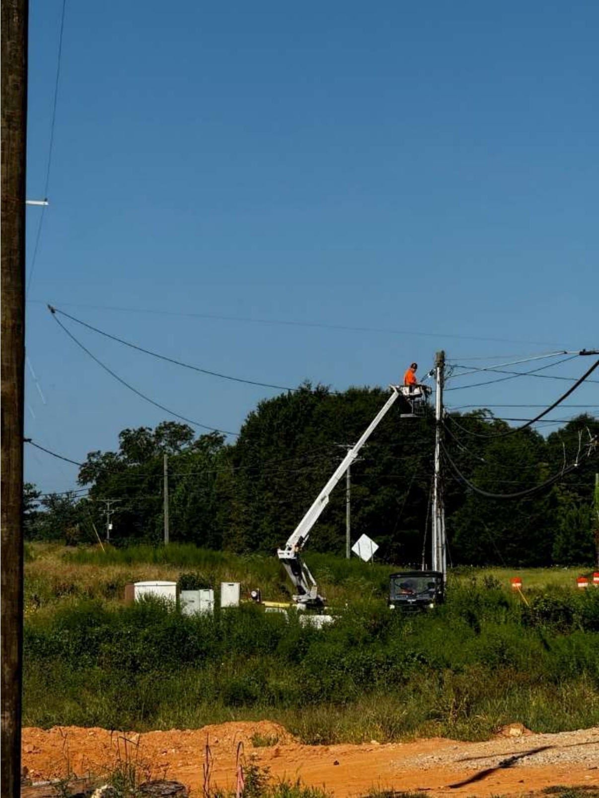
City of Monroe telecommunication crews have worked with other utilities and companies to coordinate moving telecommunication infrastructure at the appropriate times as the bypass nears completion.
