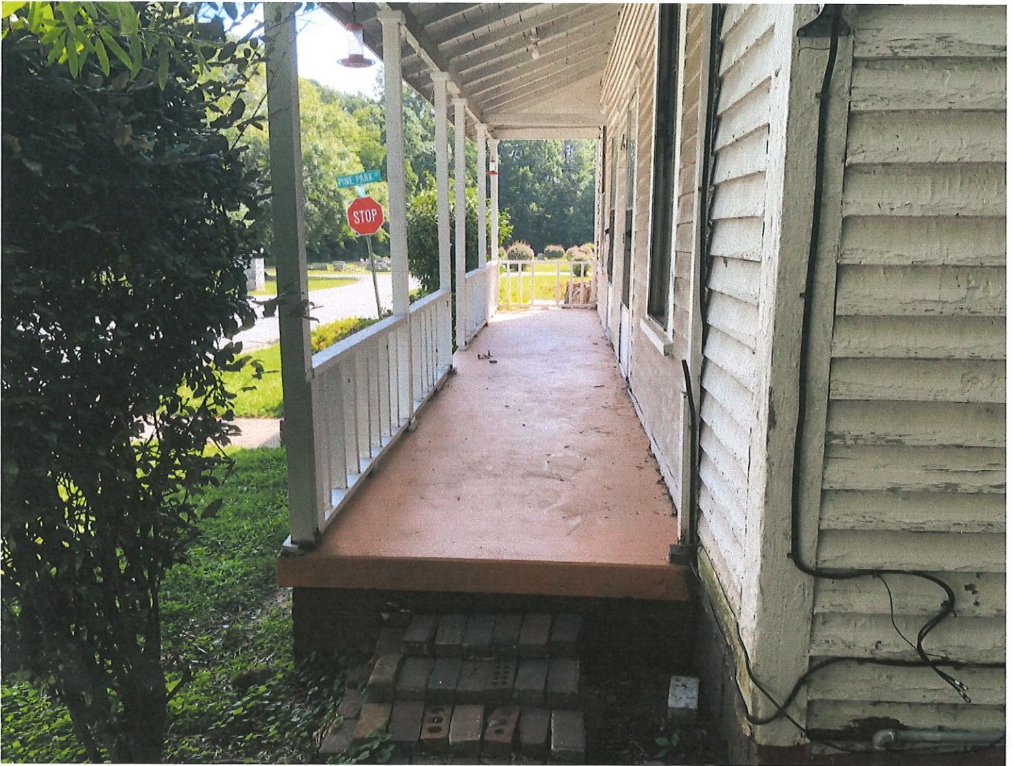
Front Porch / Missing & Rotted Railing (current) - 07/12/2019
