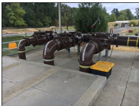
FIGURE 2.3.17 TRANSFER PUMP STATION
