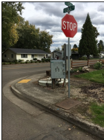
FIGURE 2.3.10 EAST 5 TH AND SOUTH COLE PUMP STATION
