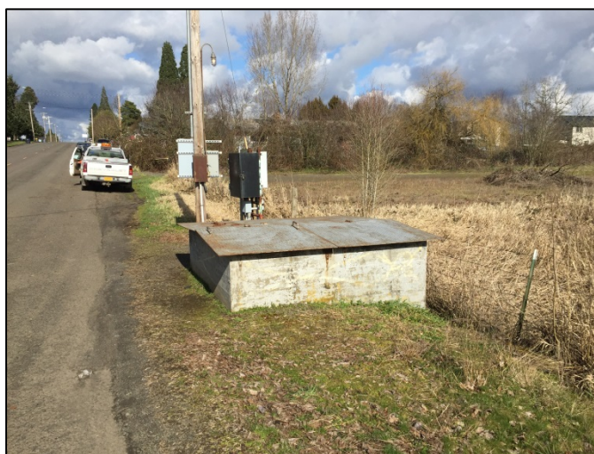
FIGURE 2.3.7 SOUTH MOLALLA PUMP STATION
