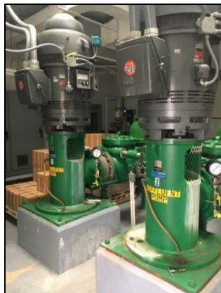
FIGURE 2.3.27 EFFLUENT PUMP STATION
