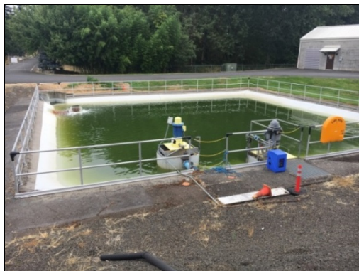
FIGURE 2.3.26 CHLORINE CONTACT BASIN
