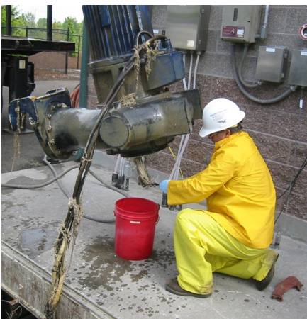
Operators take sewage pumps out of service and use hand tools to remove clogs.
