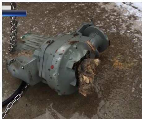
City of Bend: Pumps of All Sizes Clog with Wipes Flushed Down Toilets
