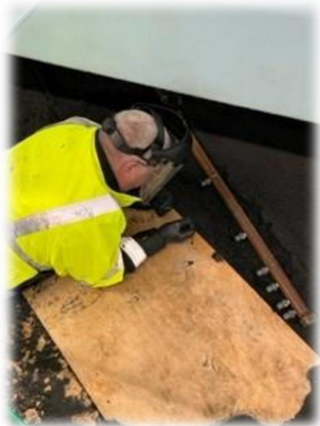
WTP Staff Works on the Trident Filters
