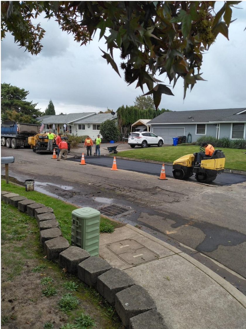
The Utility Crew dug out a section of 7 th Street, followed by paving courtesy of Jim Newman's Paving LLC
