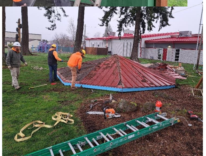
Public Works Crews Demo the Gazebo at Long Park and Reframe the Electrical Panel.
