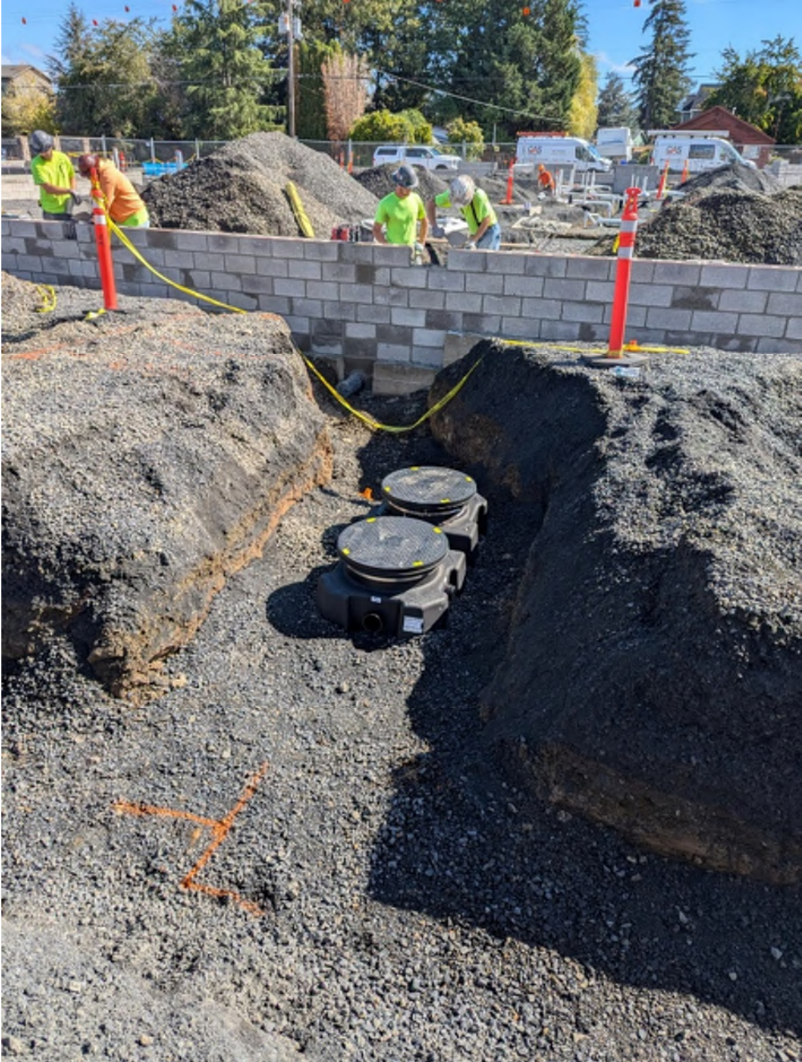
Figure 1- project grease interceptor tank system
