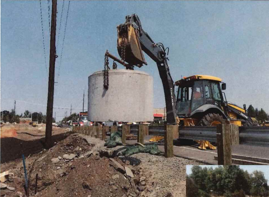
Public Works Utility Crew Adding a Section on Manhole to the Sewer Main on Hwy 213 during the Roundabout Project
