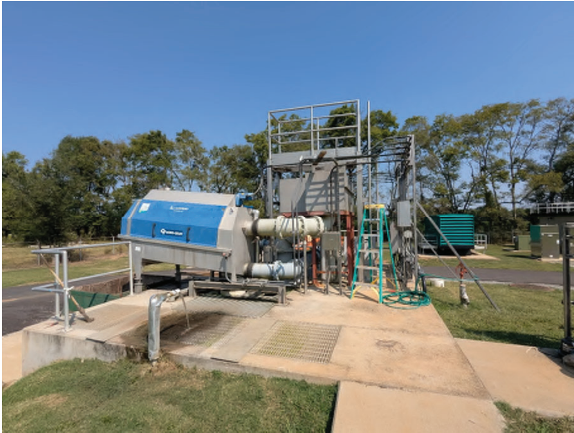
3. Headworks with fine drum screens
