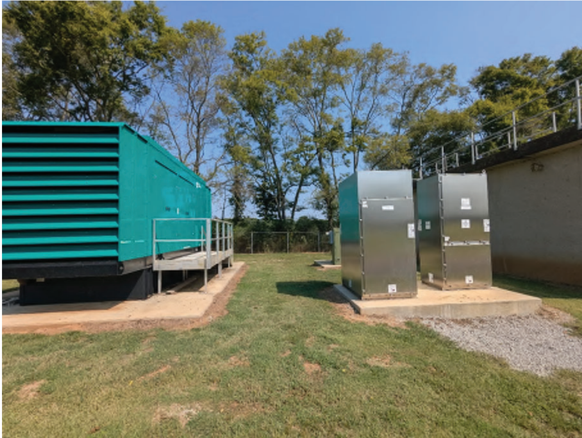
4. Generator and Automatic Transfer Switches
