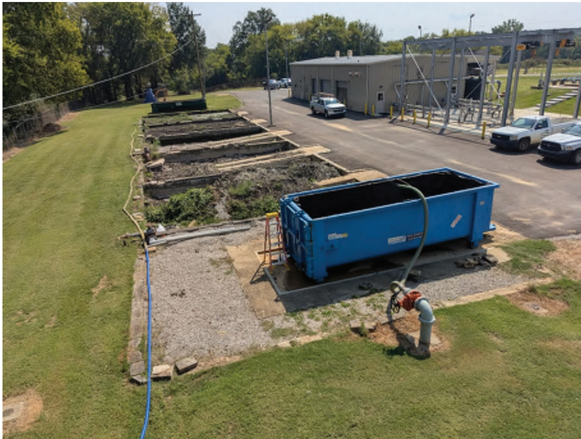
6. Sludge dewatering box and drying beds
