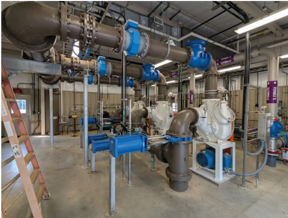
9. MBR RAS pumps
