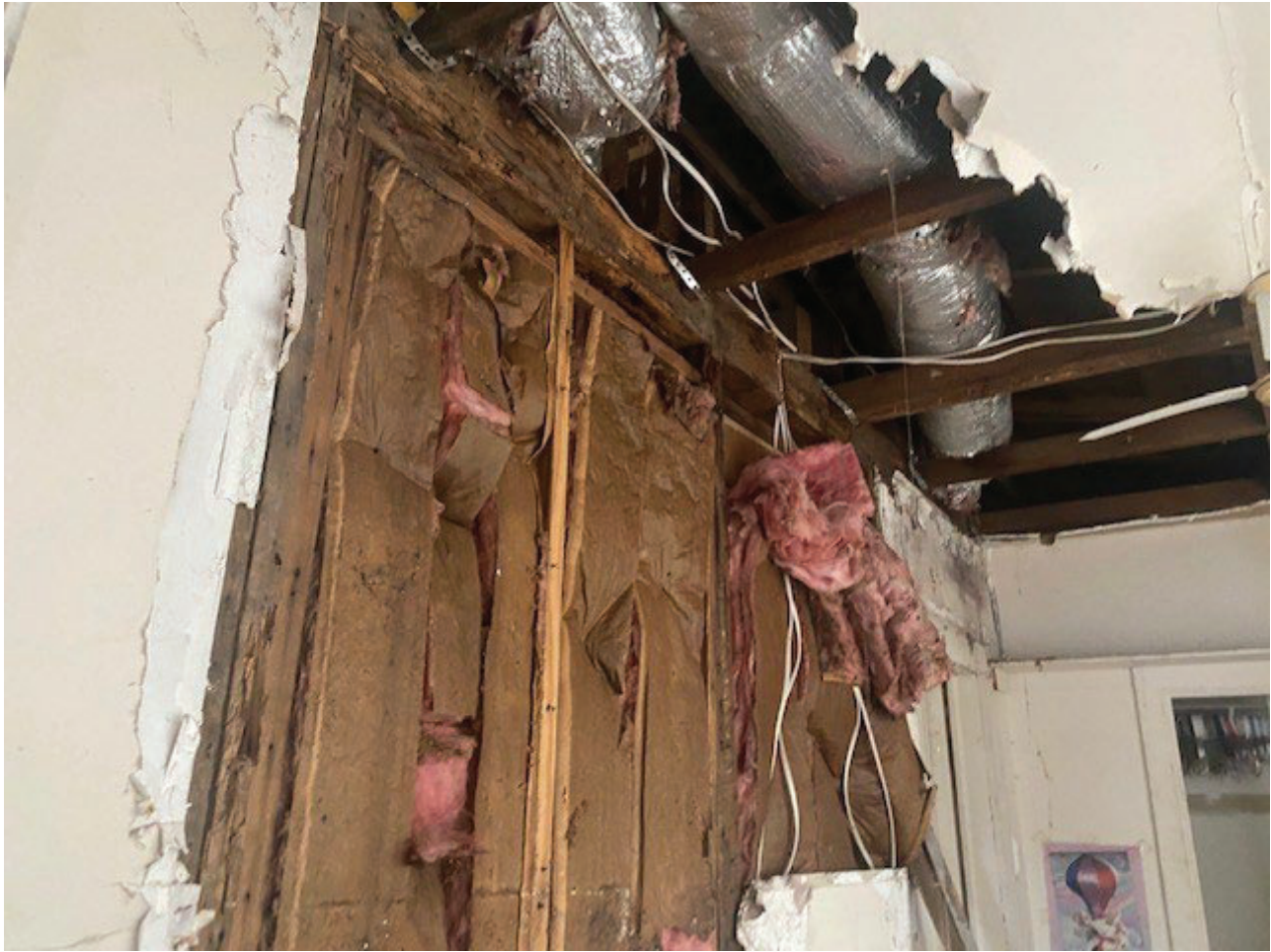
1 st Addition to the original structure. This picture shows the condition of the framing.
