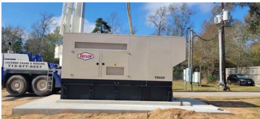
Figure 1: Newly Installed Generator January 11, 2023
