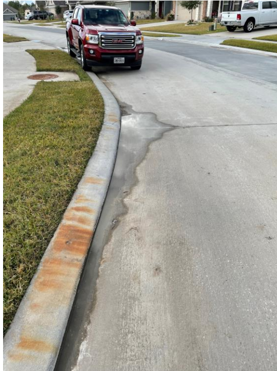
48 hours post-flooding (Before Repair)
