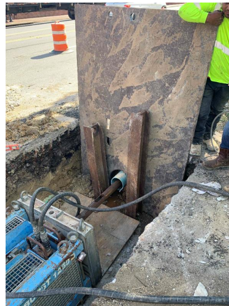
Pipe Burst at SH-105 & Cemetery St.
