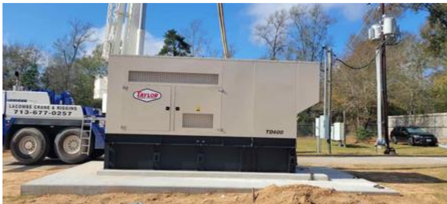
Figure 1: Newly Installed Generator January 11, 2023
