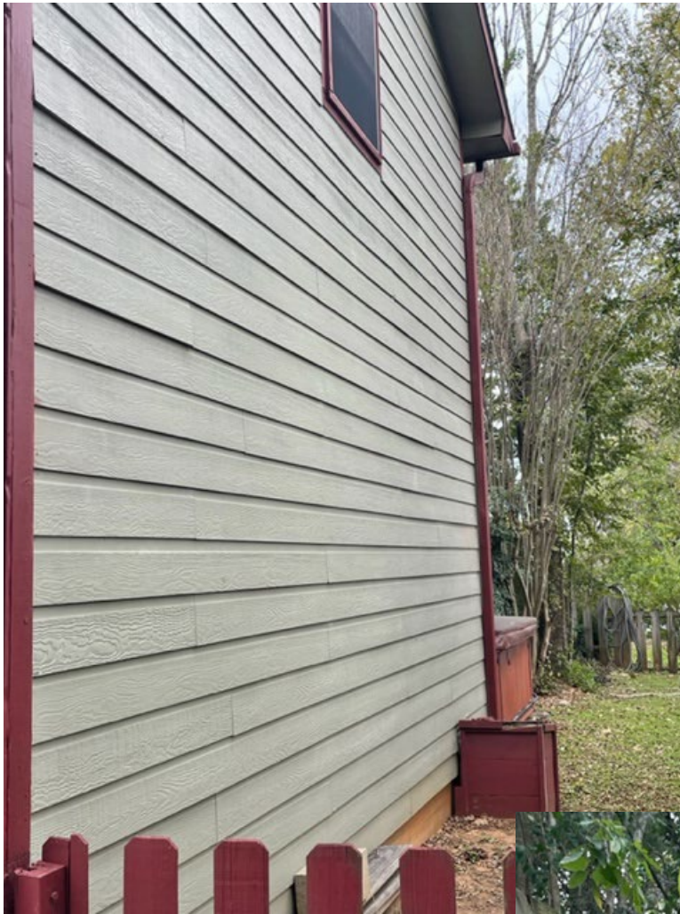
South wall of the detached garage with the hot tub from the previous photo visible. A new exterior staircase is proposed with a door to replace the window shown in the photo.
