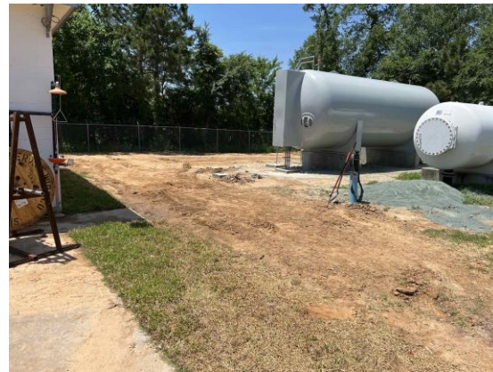
Figure 2: Hydropneumatic Tanks May 17, 2022
