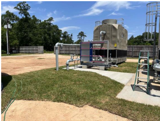
Figure 1: Cooling Tower May 17, 2022
