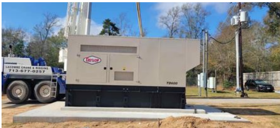
Figure 1: Newly Installed Generator January 11, 2023
