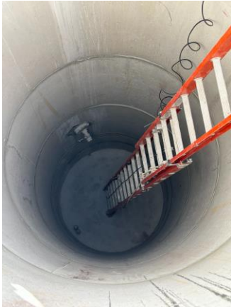
Inside Lift Station wet well January 17 th
