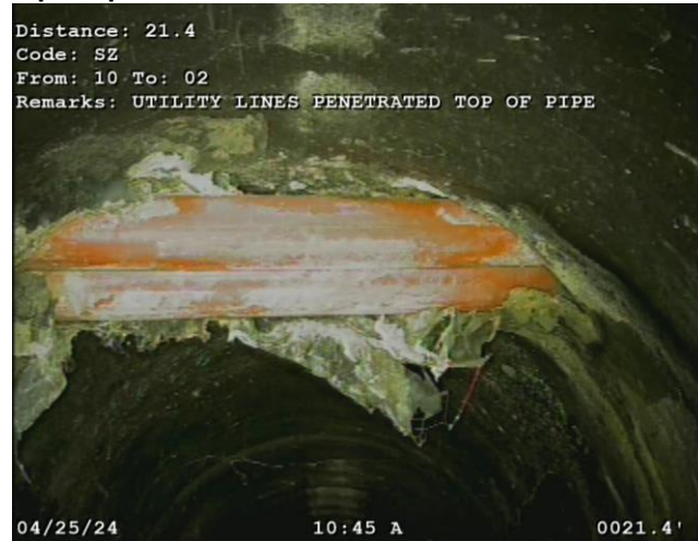
Figure 3: Utility Line Penetration
