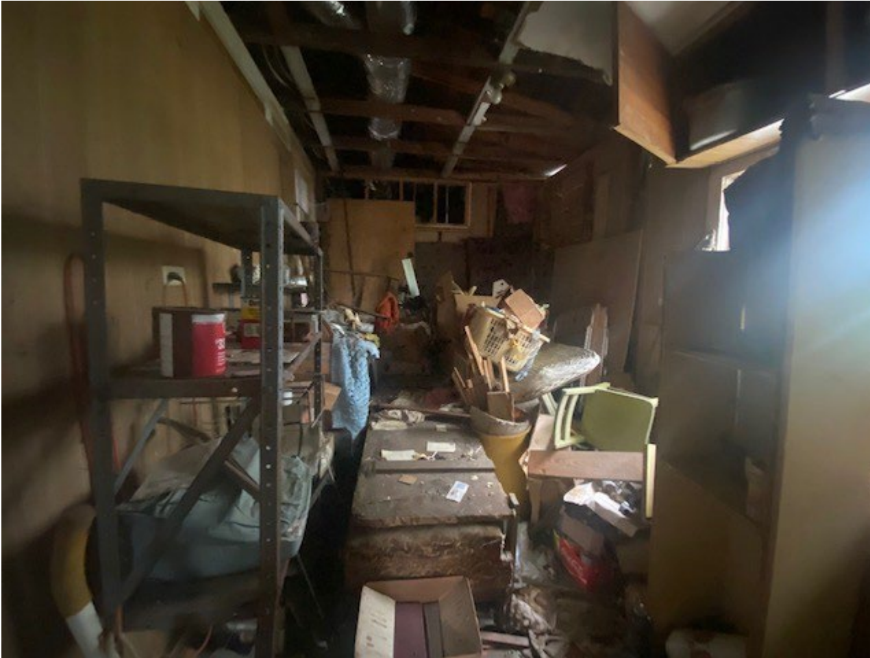
The 2 nd addition to the original home. The ceiling has fallen due to water intrusion, massive frame and subfloor damage.
