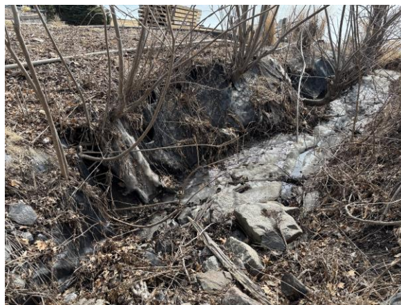
Figure 2. Erosion in the channel (looking south, Lake Minnetonka in the background)
