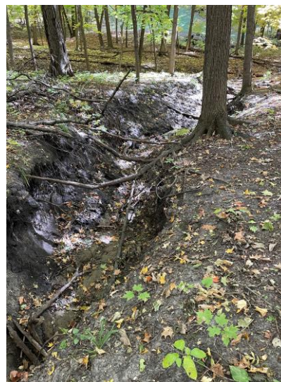
Figure 8. Erosion south of D'Chene Ln
