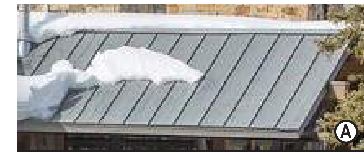
A STANDING SEAM METAL ROOF - GREY
