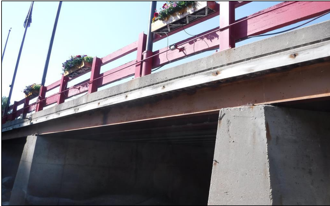
Girder 3L has heavy corrosion.
