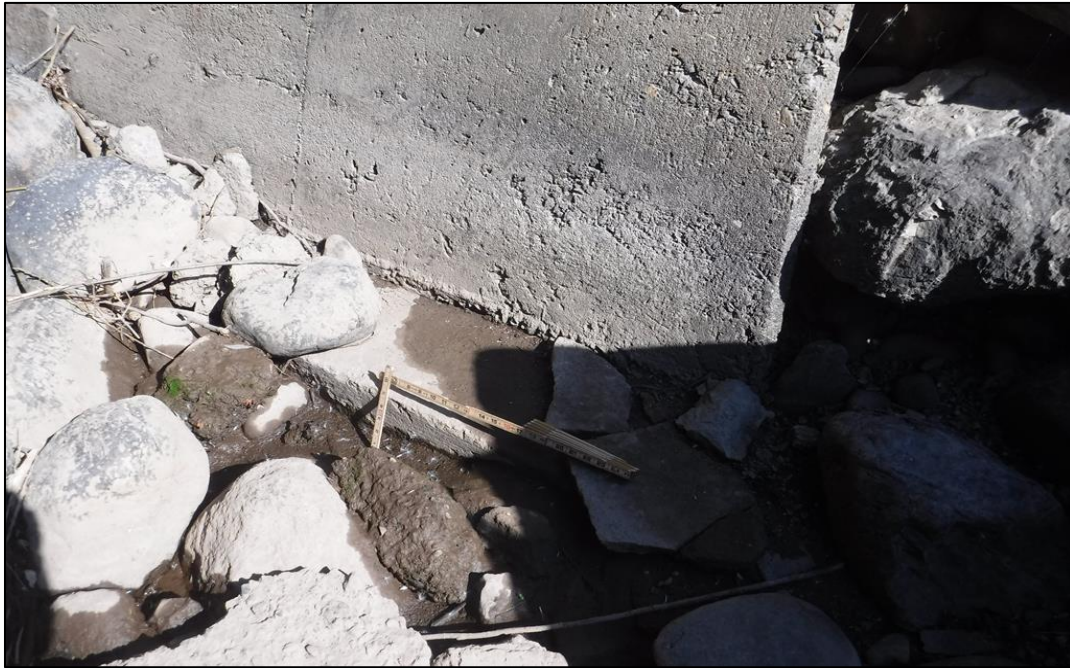
Abutment 5 exposed footing at downstream side.
