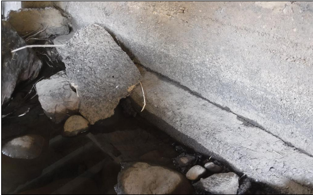
Abutment 5 exposed footing near mid length.
