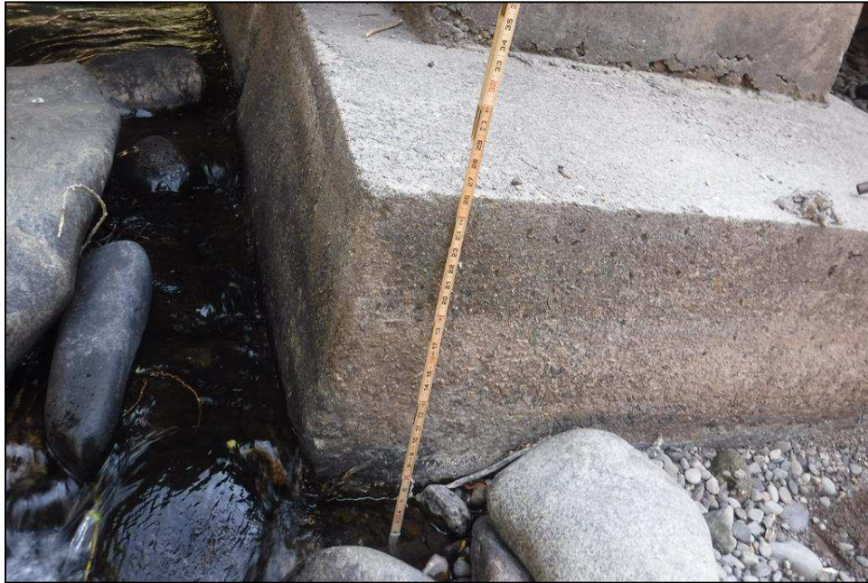
P3 exposed footing at downstream end.
