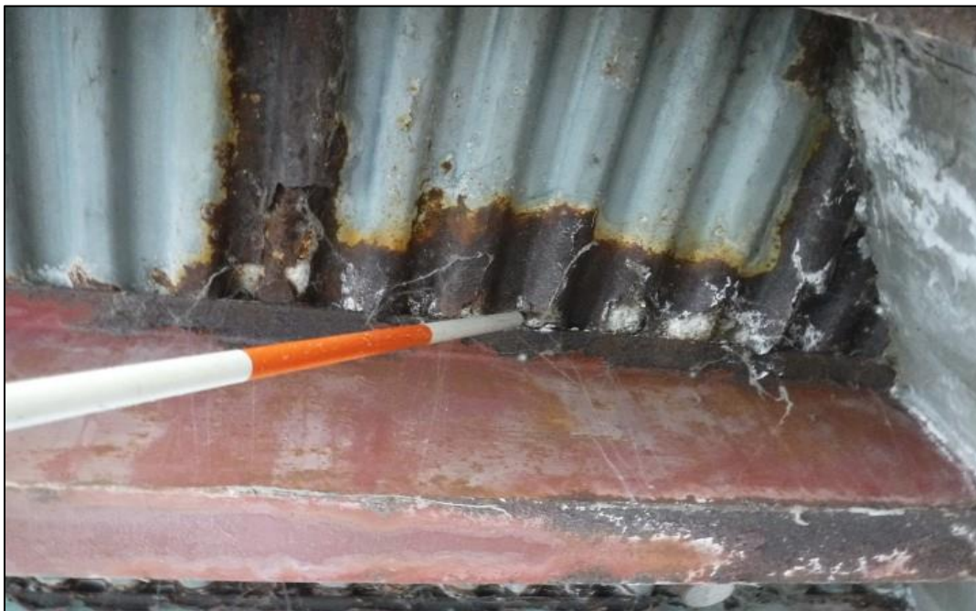
R4 rust and holes in deck forms and exposed concrete in bays 4L and 4M.
