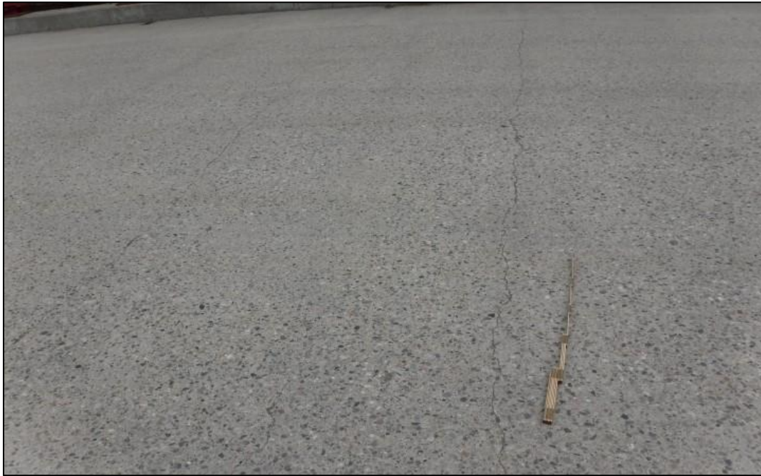
Transverse cracking and abrasion throughout deck surface.
