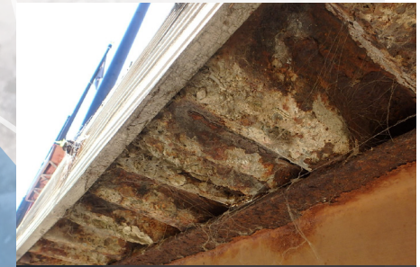
C Typical deterioration and corrosion of steel decking and bridge girders (multiple locations)
