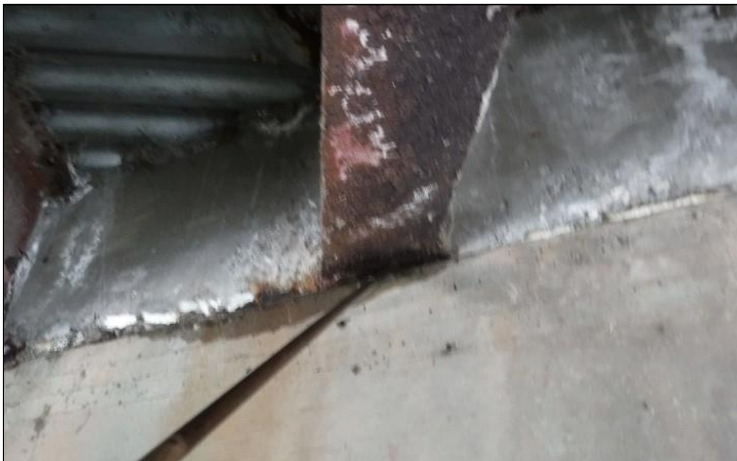
Flaking rust and section loss in bottom flanges of Girders L, M, and N.
