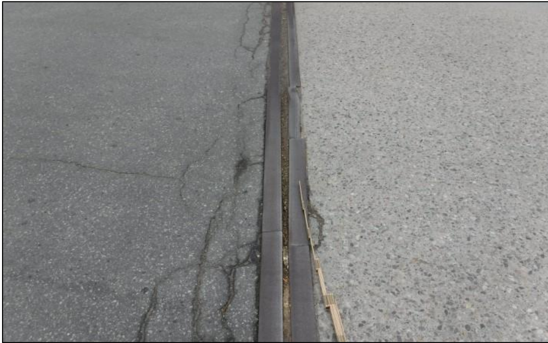
Delamination and spalls in south end of deck.
