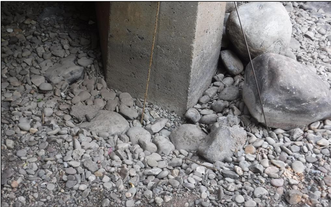
Pier 2 scour at downstream side (2 of 2).
