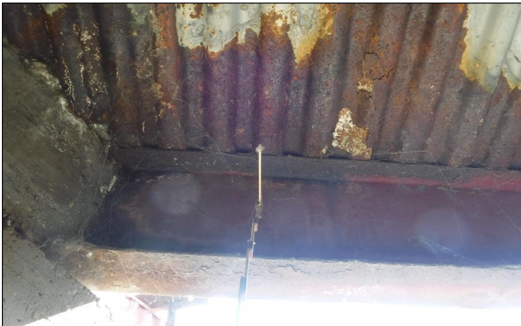
Metal deck at Bay 4N has corrosion.
