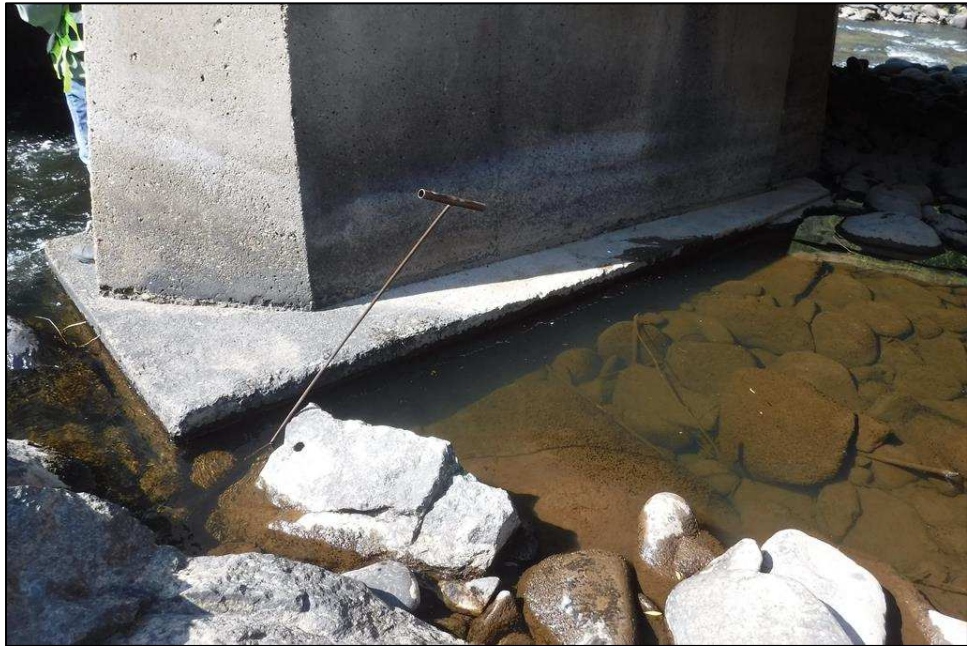
P4 north side exposed footing.
