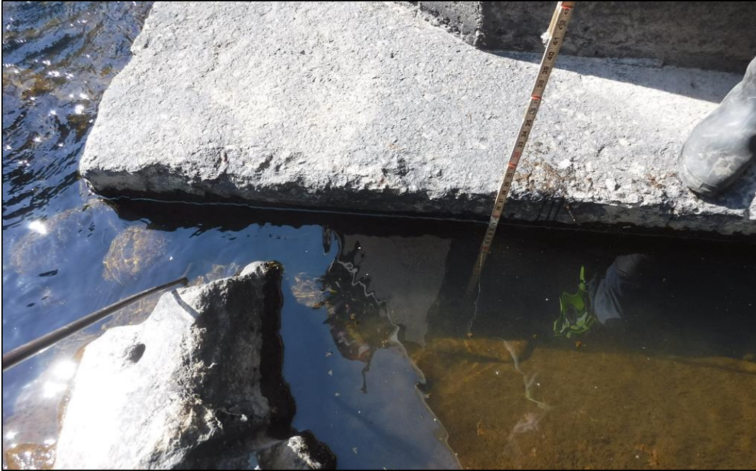
P4 exposed footing at northwest corner.
