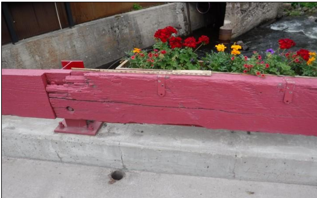
West timber rail broken plank.
