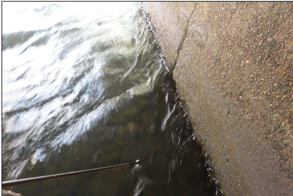
P3 south side undermined footing at upstream end.
