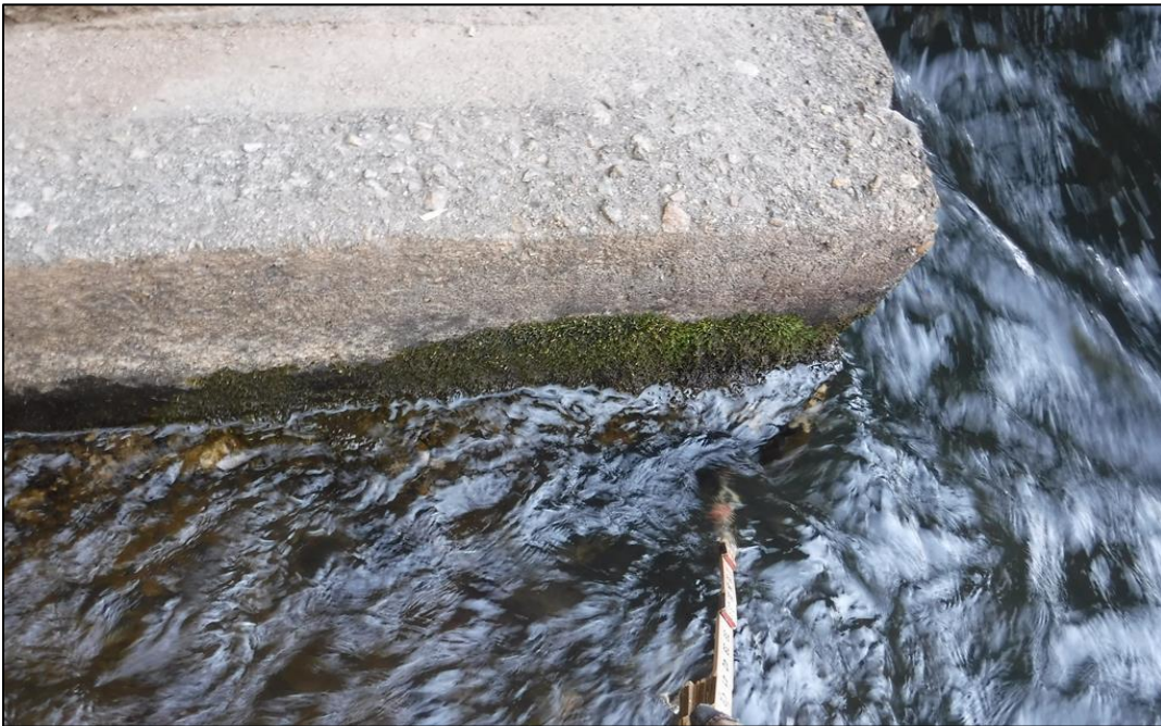
P4 undermining at SW corner upstream side.
