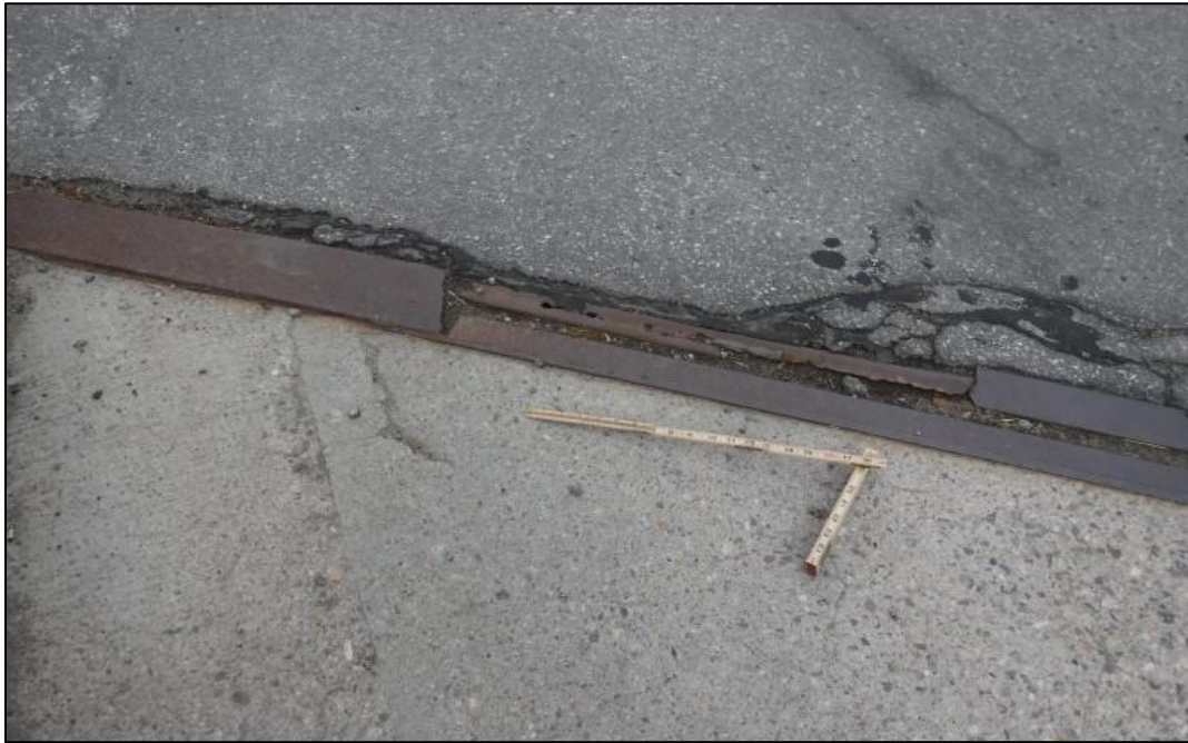
Cover plate missing and rust holes in armor angles at S joint near E curb.
