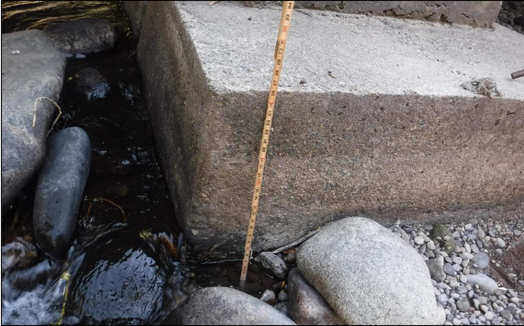
P3 exposed footing at downstream side.
