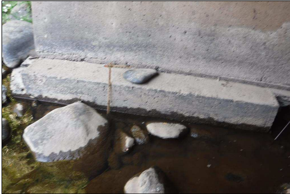
Abutment 5 exposed footing.
