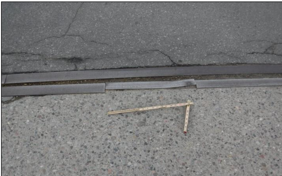
Damaged joint angle at south joint near centerline of roadway.
