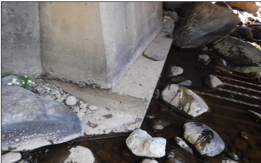
Abutment 5 exposed footing at northwest corner.
