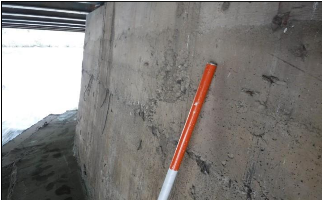
Honeycombs at Pier 2.
