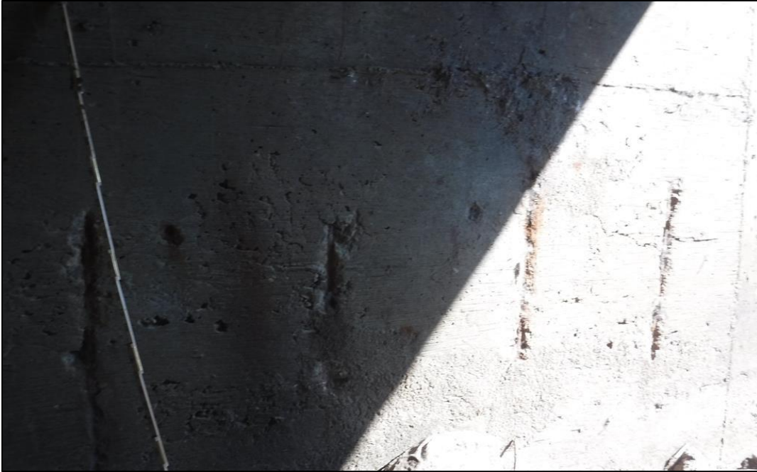
Abutment 5 has 5 locations of exposed rebar.
