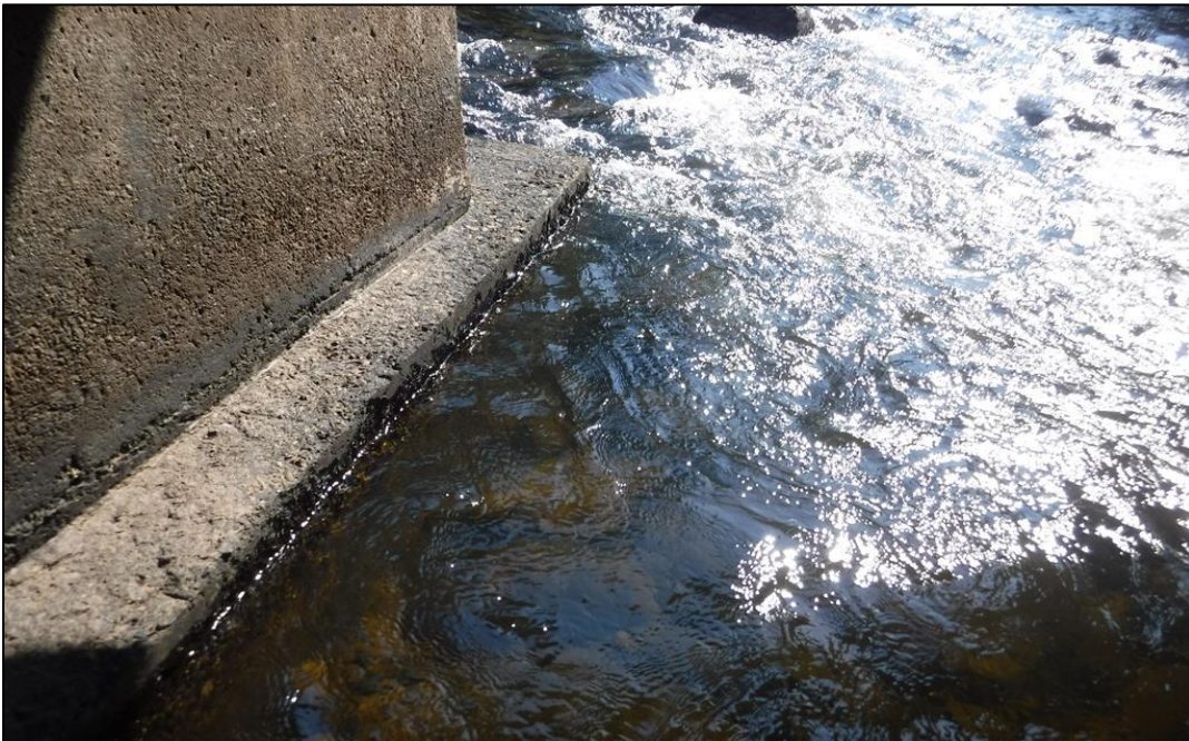
P4 exposed footing at south side.
