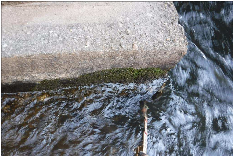
P4 southwest corner undermining at upstream end.
