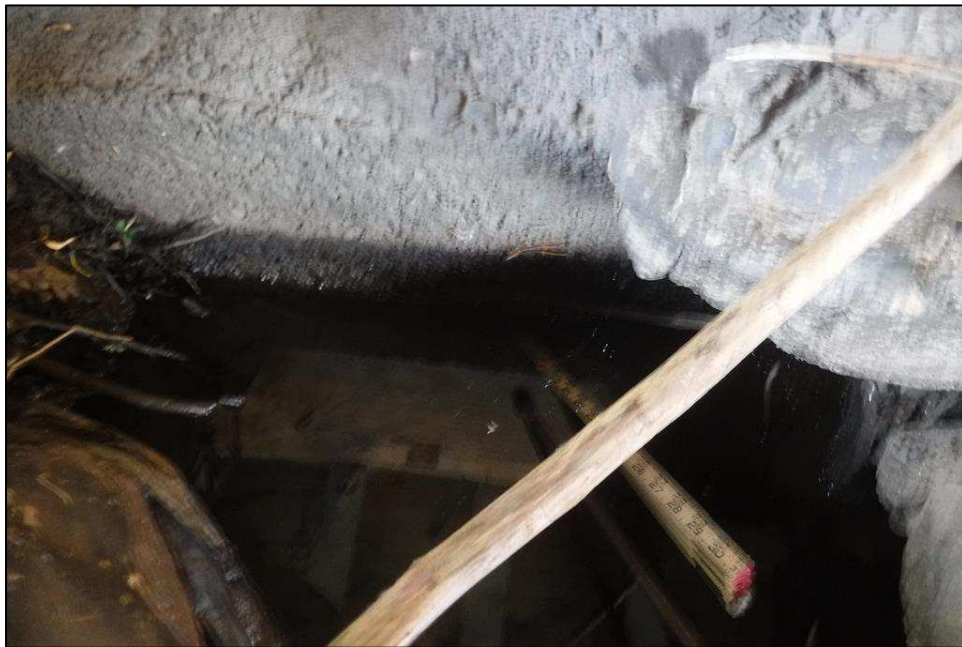
Abutment 5 undermining at mid-section.
