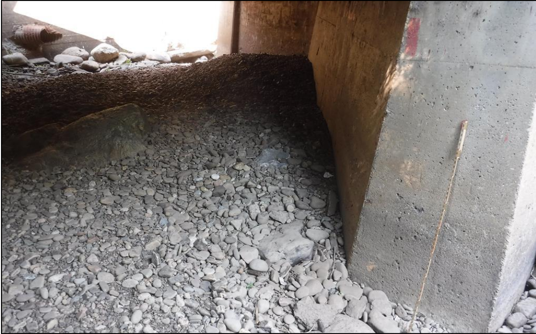
Pier 2 scour at downstream side (1 of 2).
