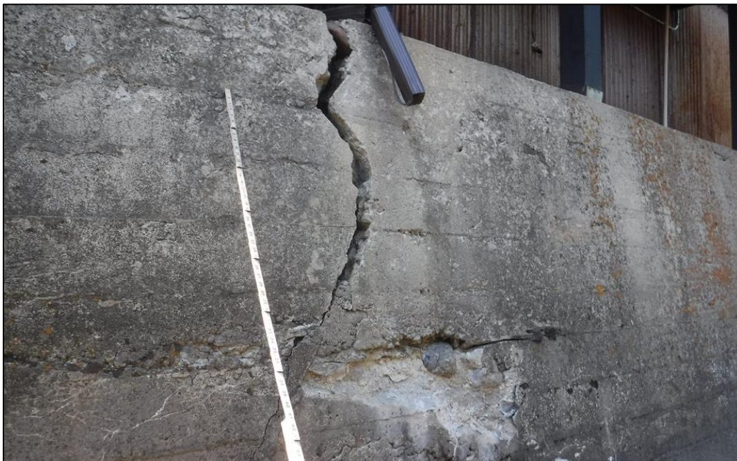
SW retention wall vertical crack.
