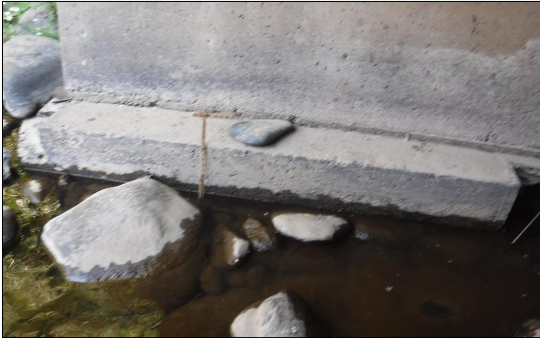
Abutment 5 exposed footing at north end (upstream).
