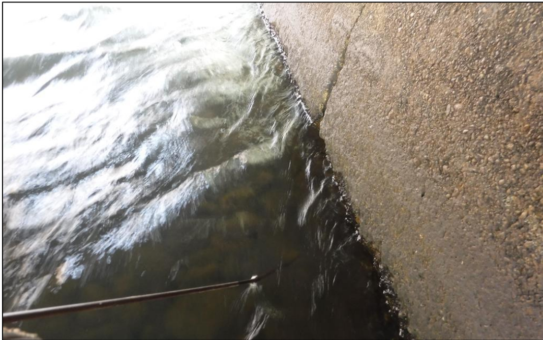
P3 undermined footing at upstream south side.
