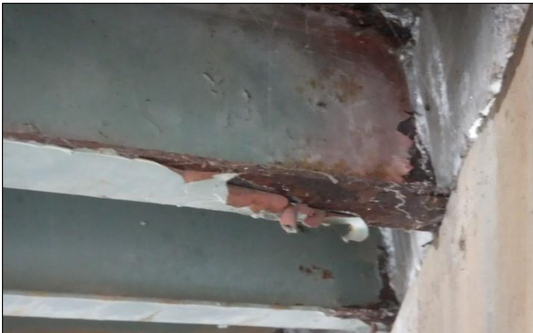
Failed paint on ends of girders (Typical girders A-K).
