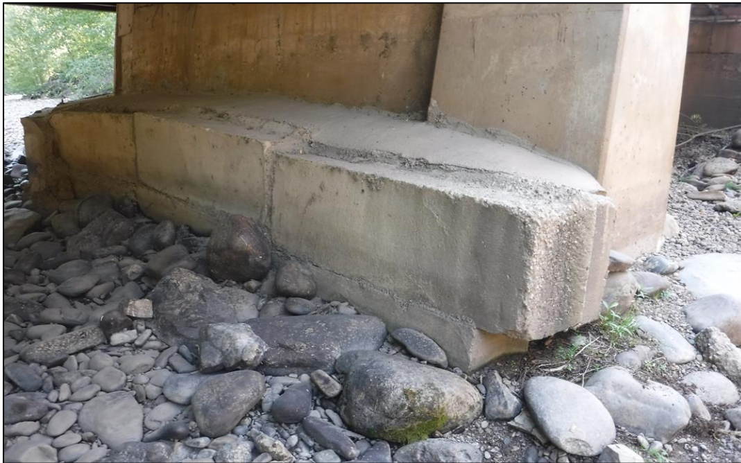
Scour around Pier 2 footer (2 of 2).
