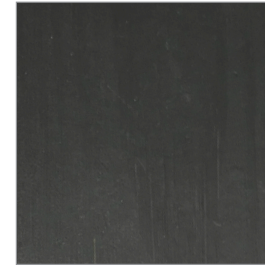
Soffits, Fascia & Railing Stained Concrete
