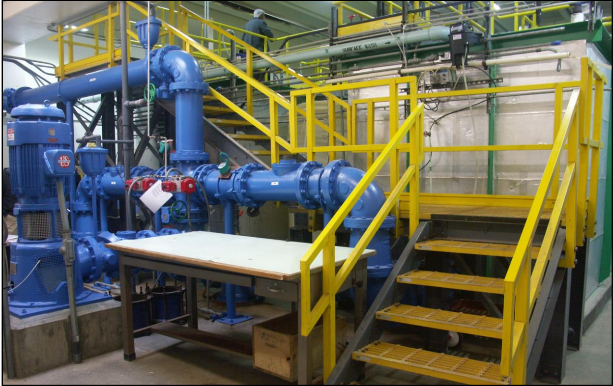
Figure 6. Example Packaged Treatment Units. Breckenridge, CO.
