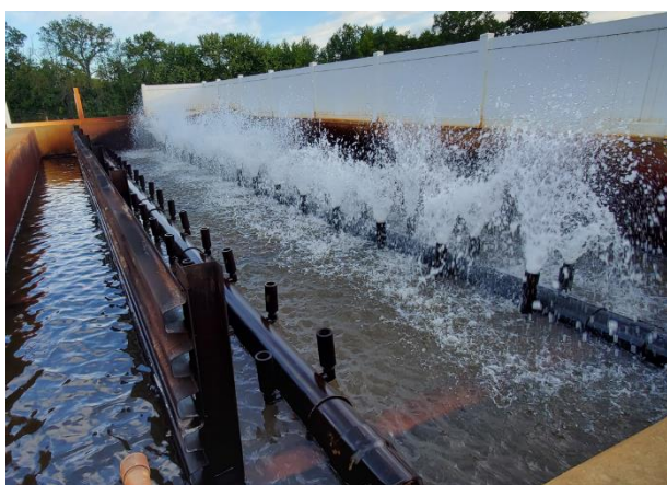
Figure 11. Example of Fountain Aeration of Iron
