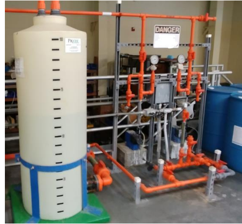
Figure 7. Example Coagulant Feed System
