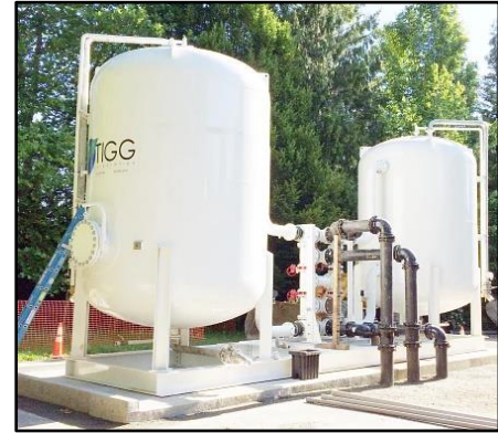
Figure 8. Pressure Filter Tanks for Adsorptive Inorganics Removal
