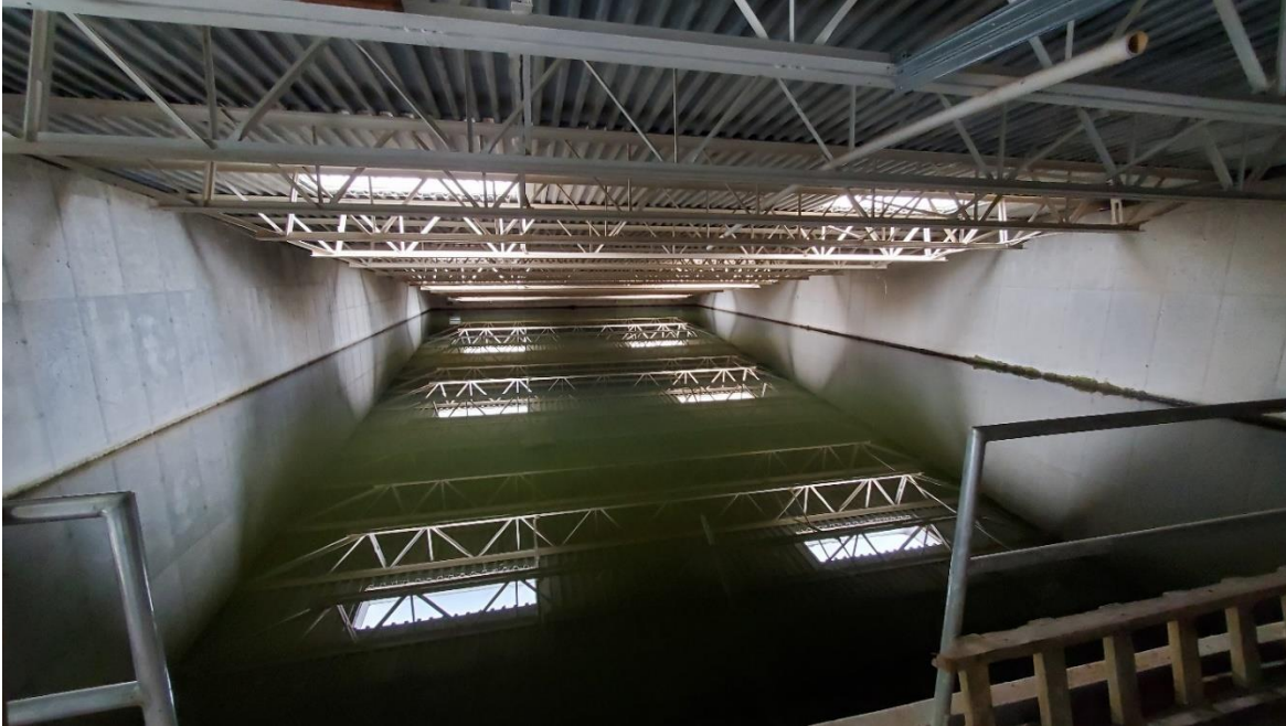
Figure 4. Minturn's Existing Slow Sand Filter (Filter 3)
