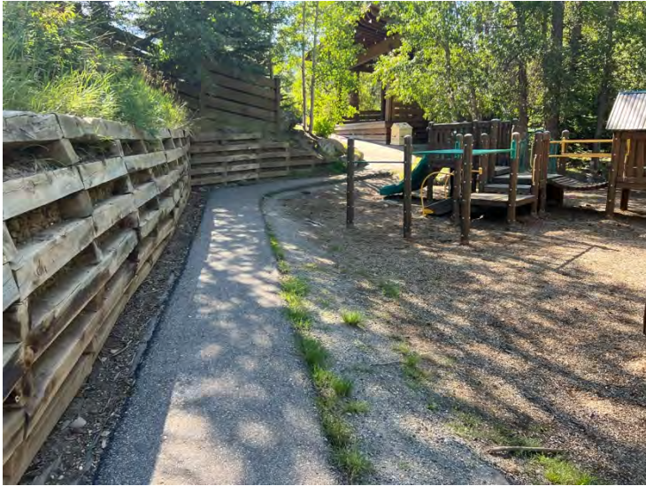
Failing Retaining Wall, Playground, and Interior Driveway
