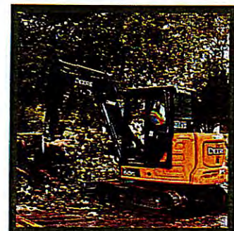
Downed / Hazardous Tree Removal
