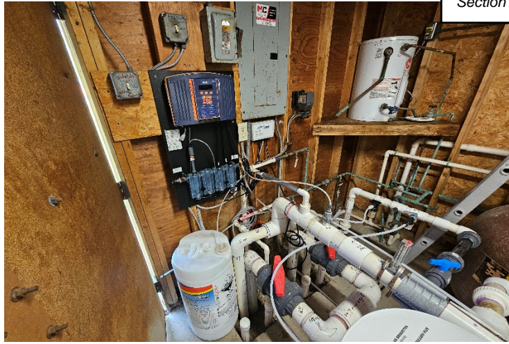
Figure 4: Tank Hot Water Heater and piping
