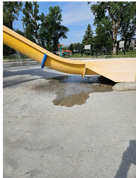
Figure 2: Joint leak below slide.
