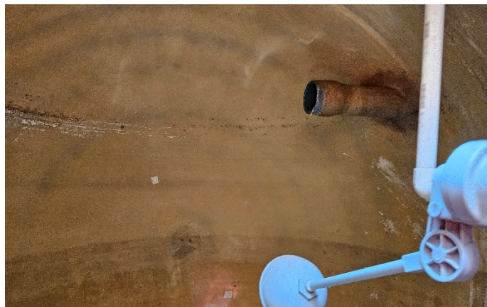
Figure 5: Scum line on tank walls at overflow pipe penetration.
