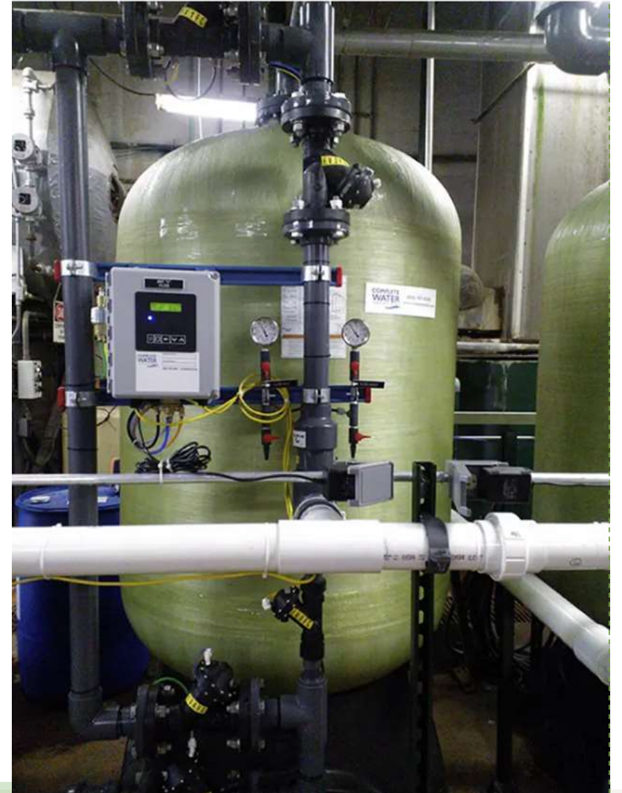
Typical Greensand Filtration Unit Source: Complete Water Solutions
