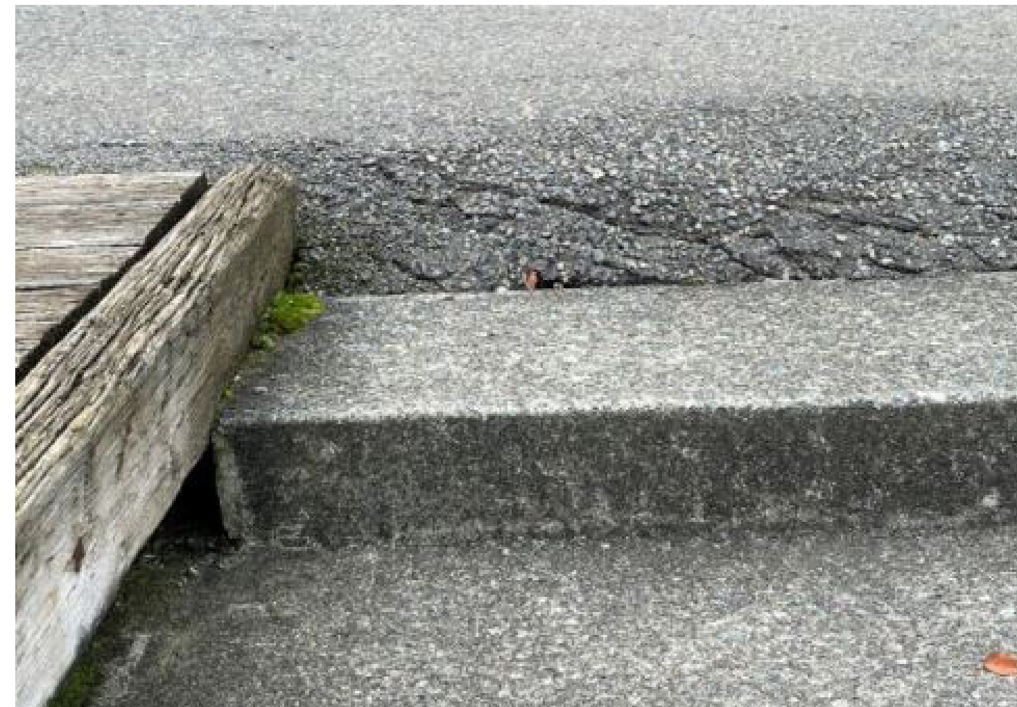
6" of settlement at south steps
