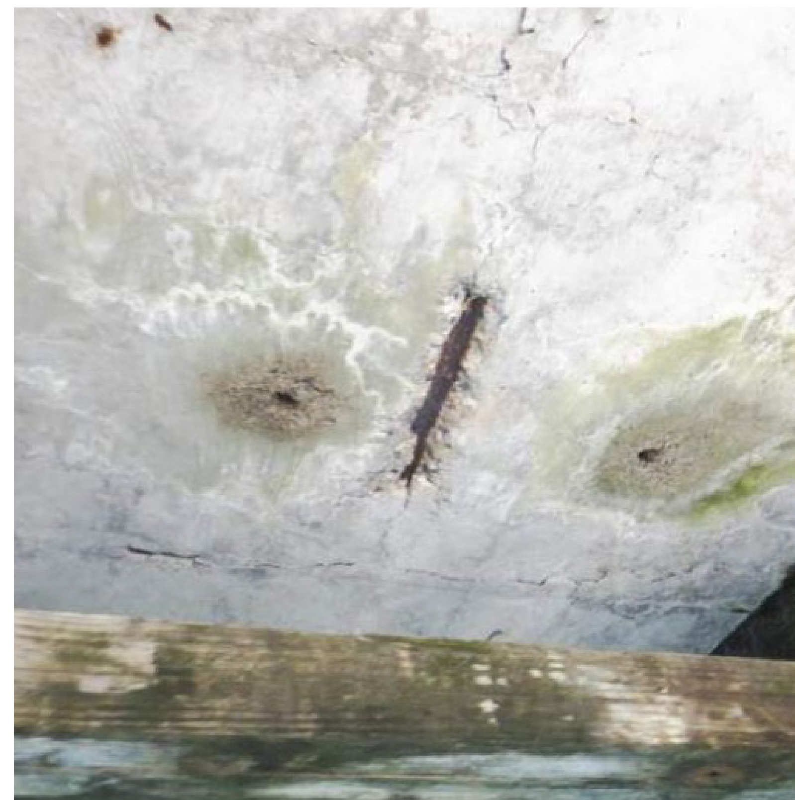
Delaminated, spalling reinforcement
