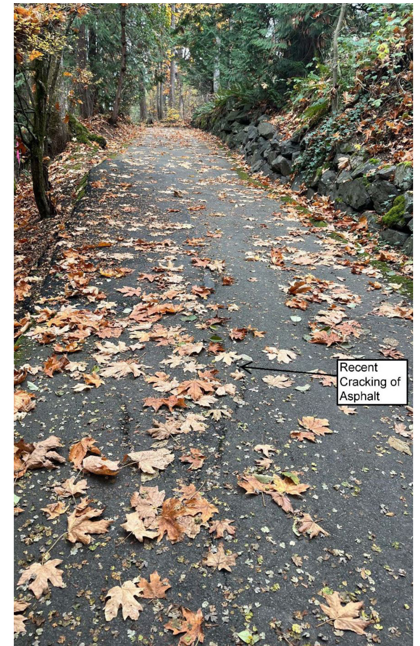
Recent cracking of asphalt
