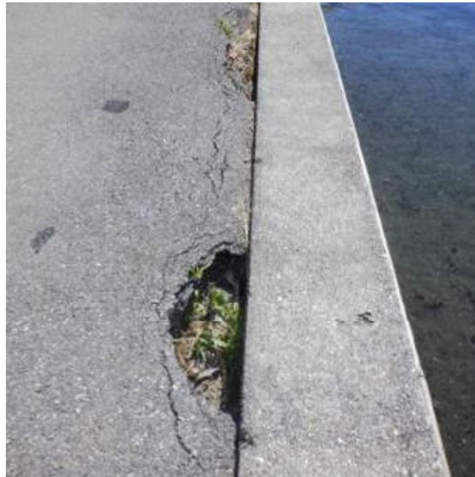
Sinkholes on swimming pier
