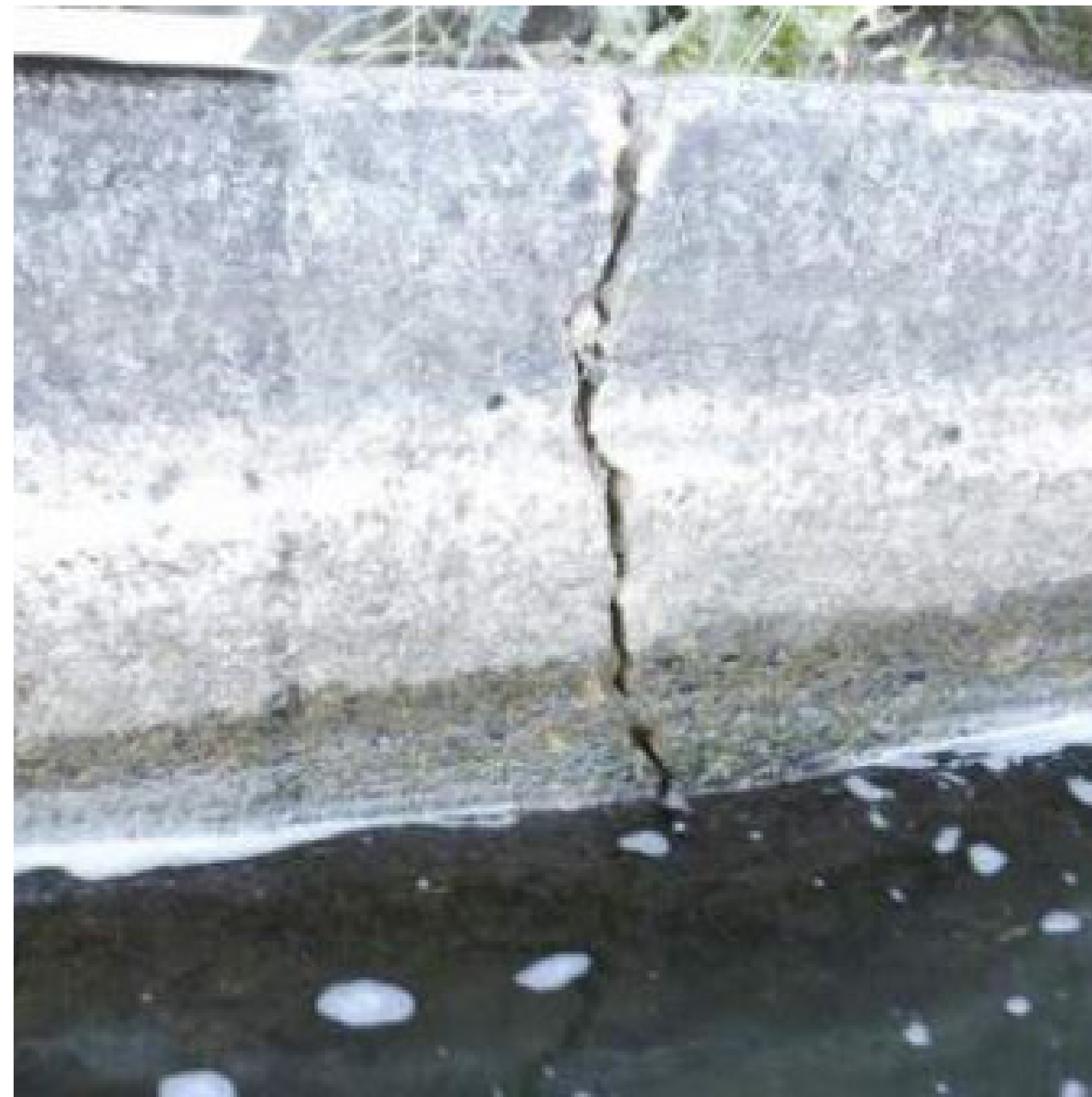
Cracked concrete bulkhead
