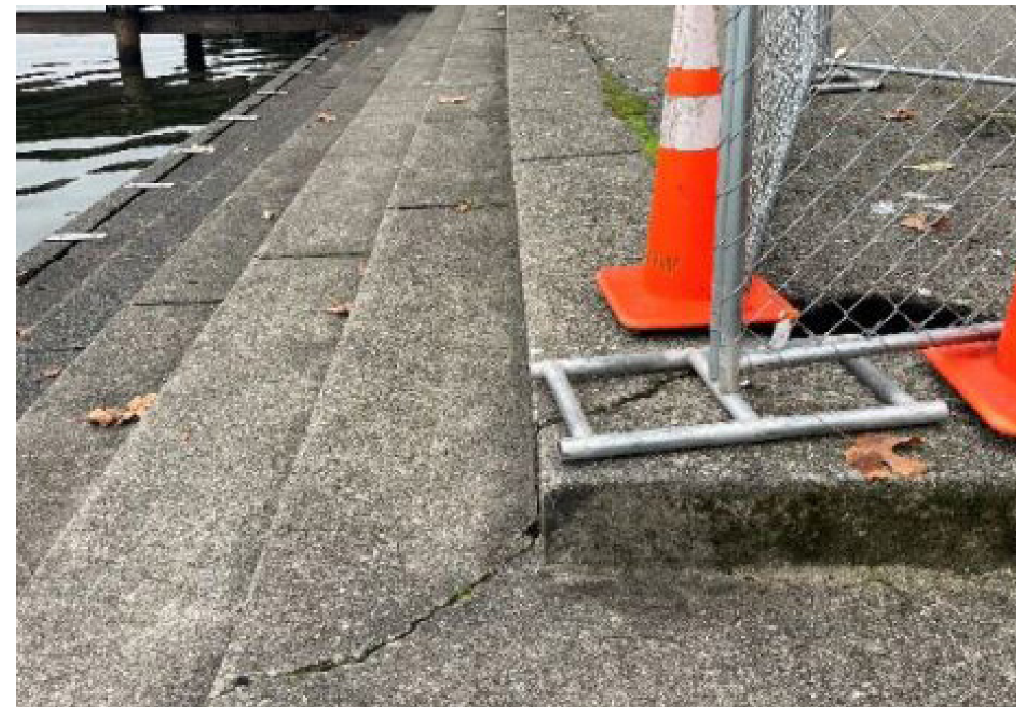
Cracked concrete stairs & sinkhole
