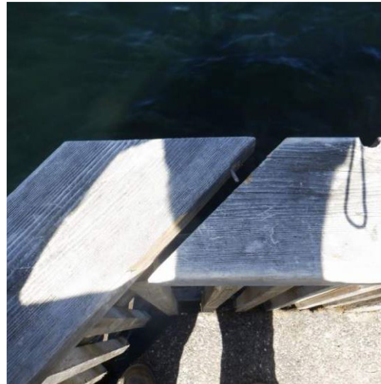
Failed railing connection
