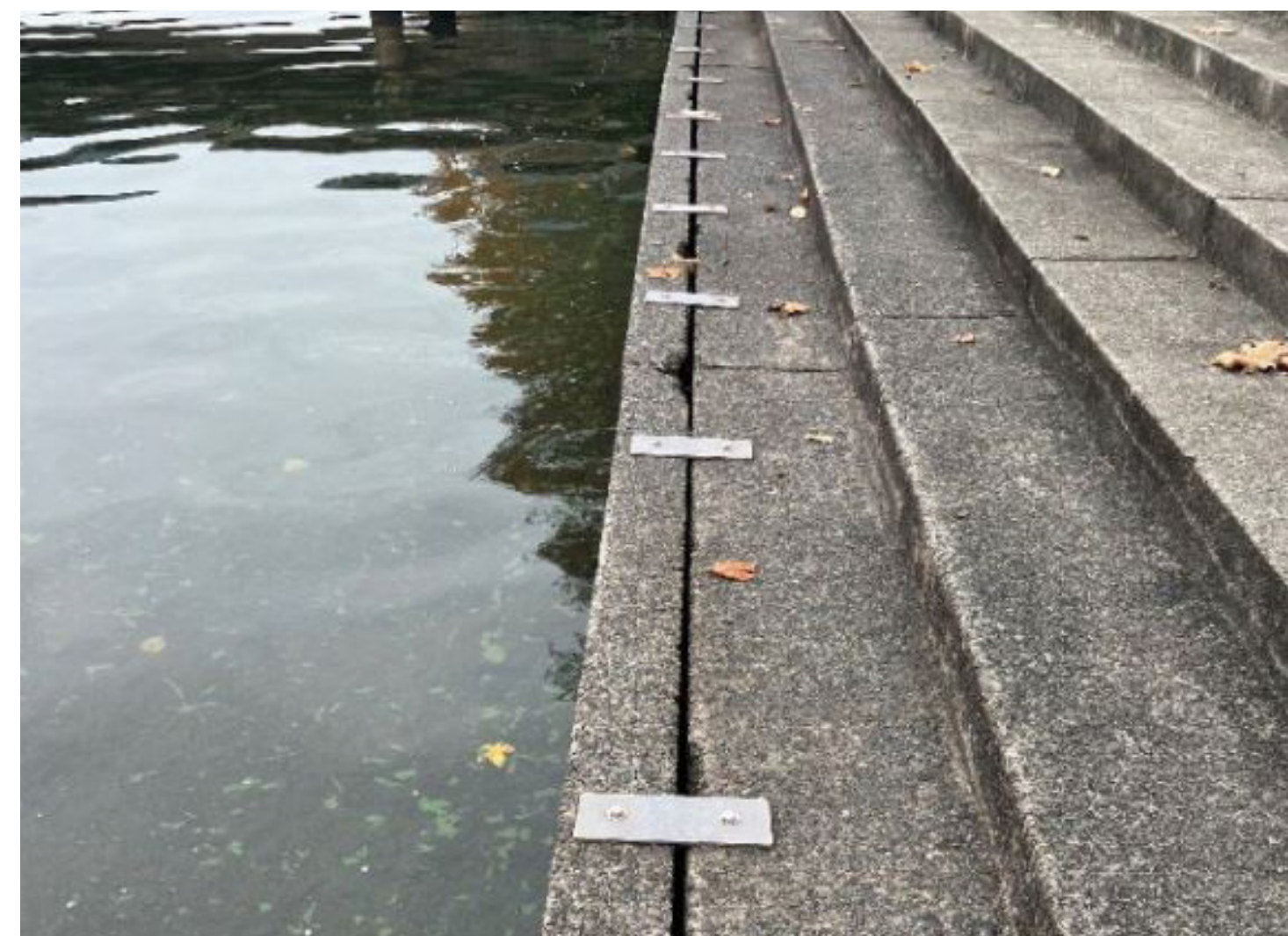
Facade separated from steps
