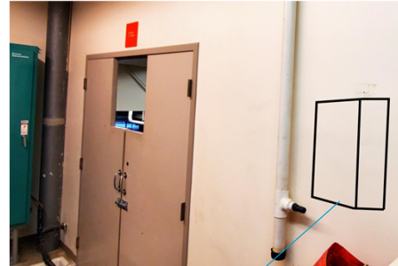
NEW PLC PANEL LOCATION
