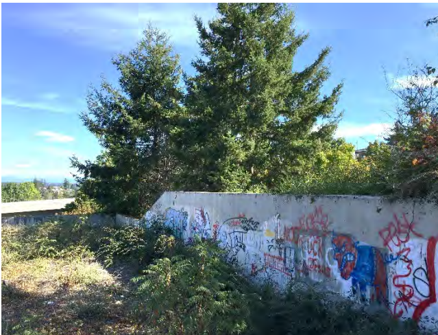
WSDOT Maintenance building rooftop – walls with graffiti.
