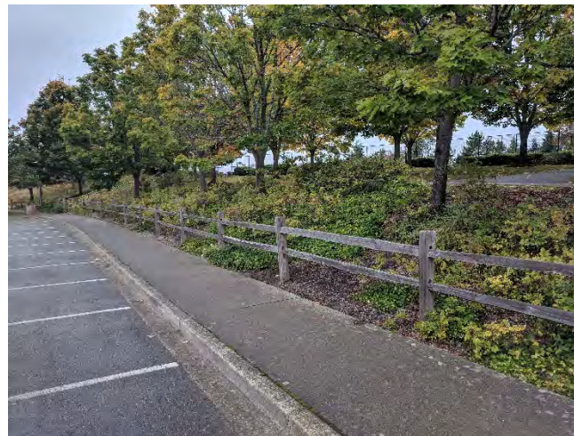
Trees, shrubs and groundcovers all display signs of declining growth. Remove all vegetation and improve soil with scoop and dump method.
