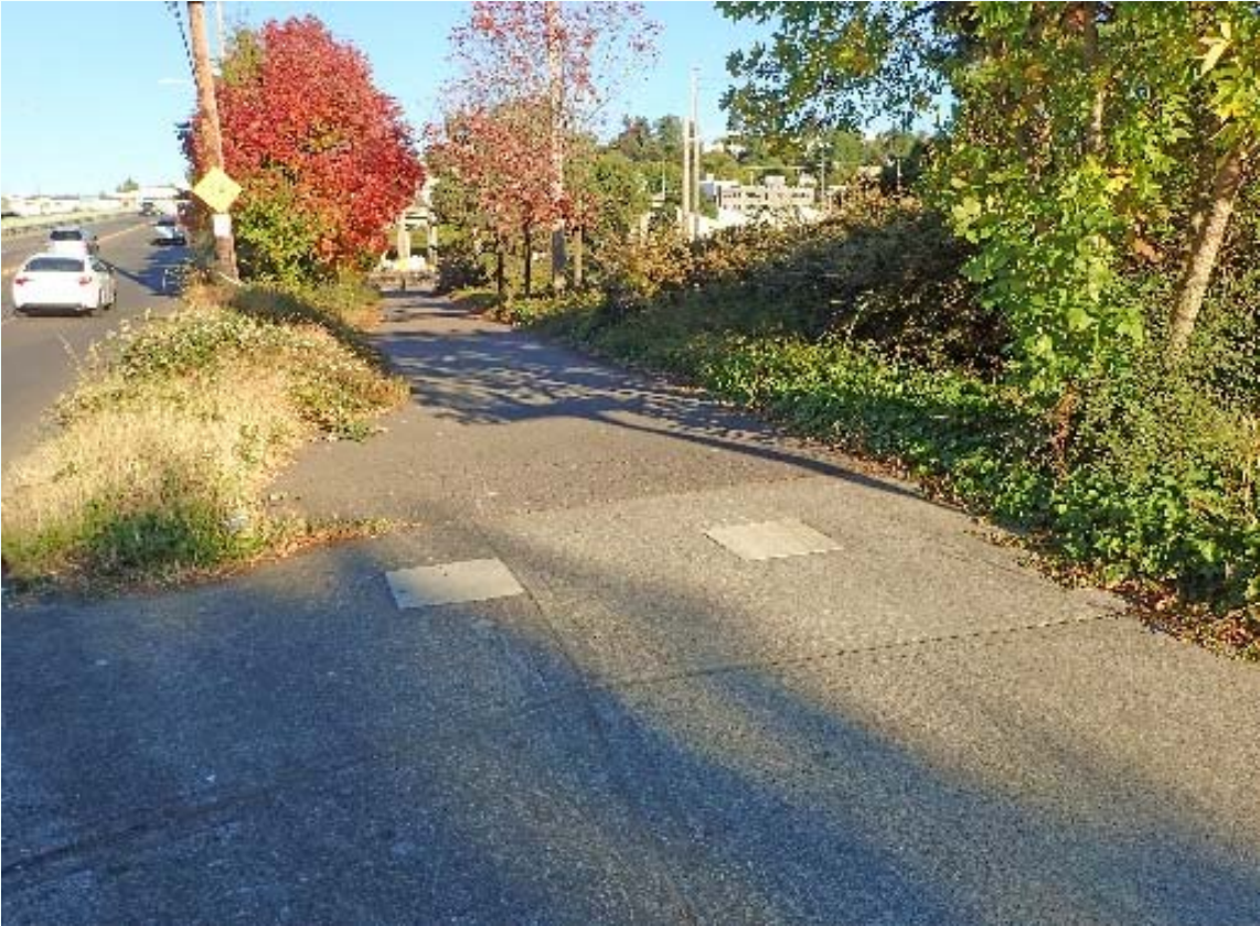
At locations where bollards are removed, the existing bollard and any in-pavement structural support should be removed in their entirety and replaced by a full repair patch. The repair patch should be a continuous surface with the surrounding trail surface.
